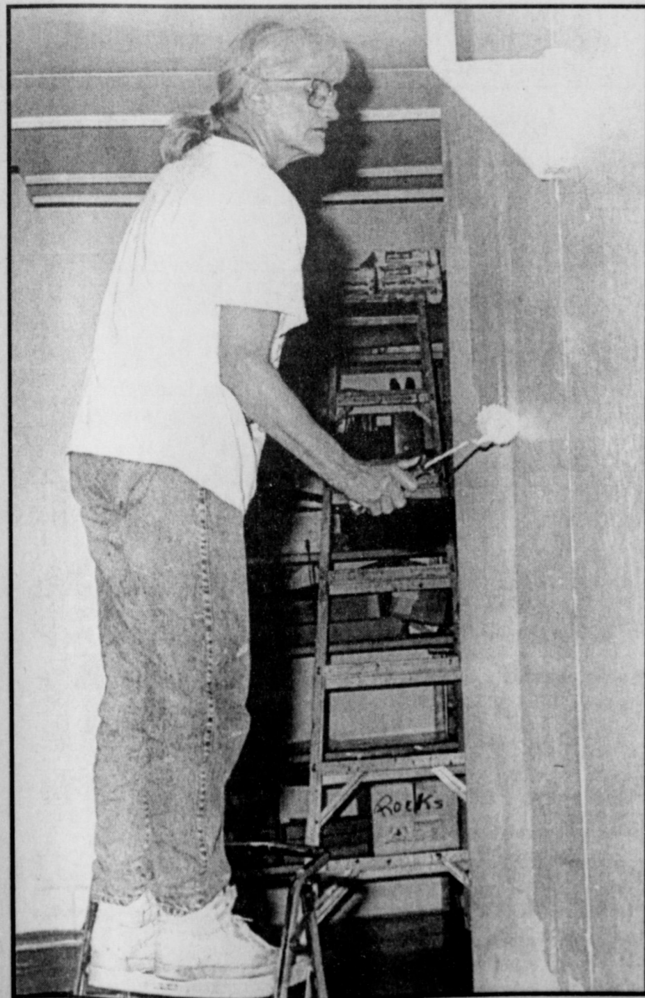
FINAL TOUCHES are underway for the Aug. 17 opening of Iowa Park schools. Thena Richardson is shown here applying a coat of fresh paint at Bradford Elementary.
