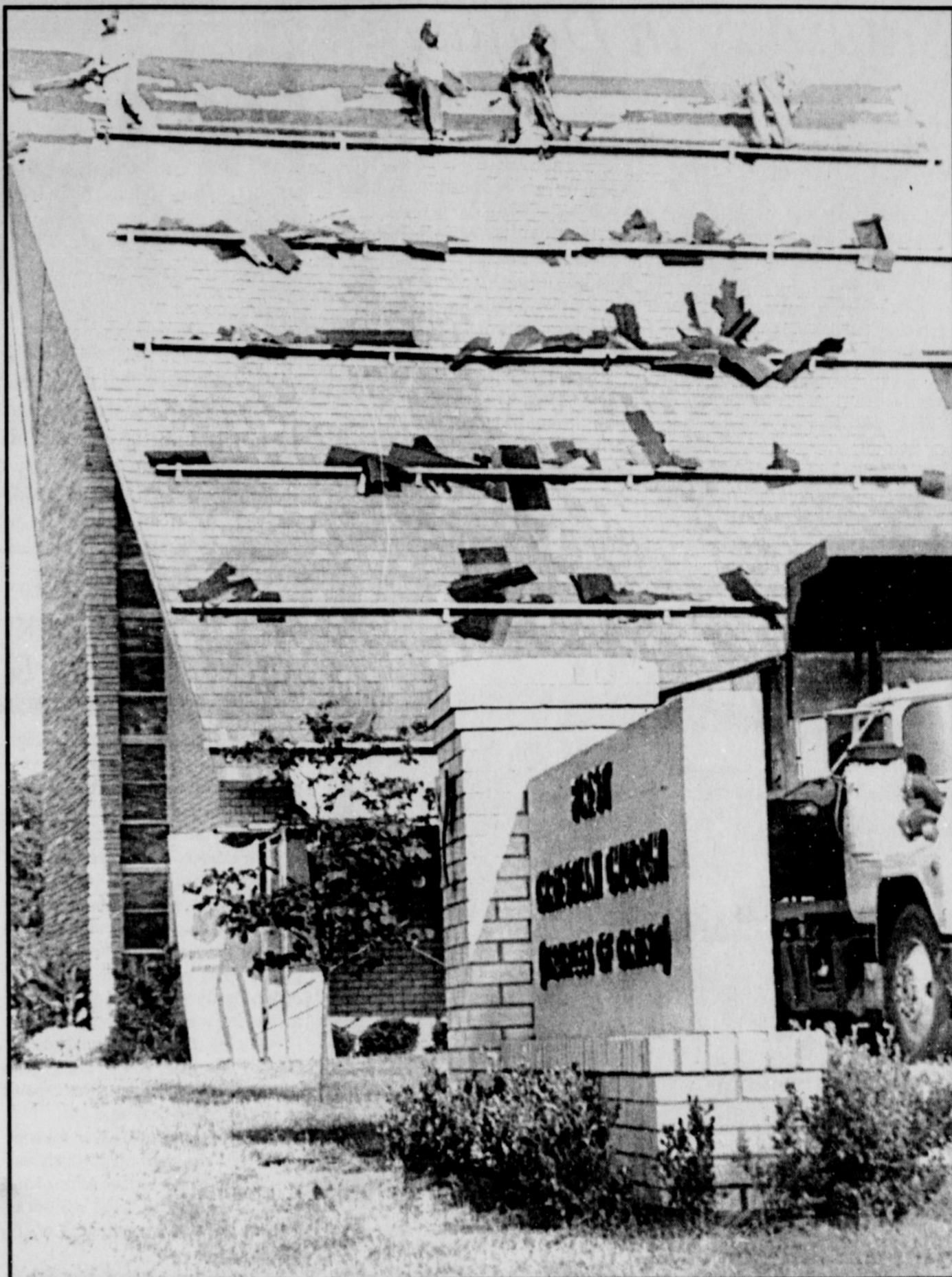
WORKERS HOT ON THEIR JOBS - A roofing crew began stripping off the roof Monday morning of First Christian Church. They had covered the stripped area with tar paper before the rains began late that afternoon.
