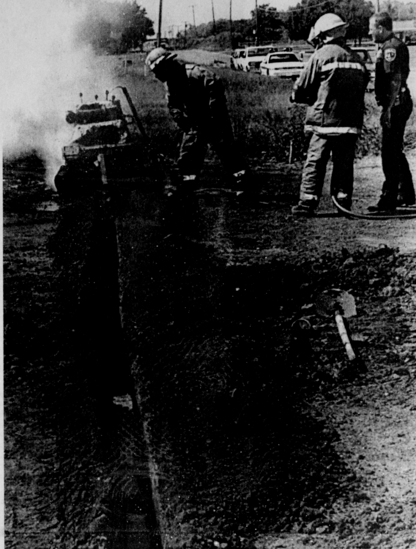
CLOSE CALL - A fire erupted Tuesday morning in the front yard of 1615 Johnson Road, when a ditching machine cut into a natural gas line. T.J. Bean, the operator, said he was digging a ditch for a yard sprinkler at the time. He said he had been assured by a Lone Star Gas representative that the line was deeper than the 10 inches he was digging. He shut down the machine, which was totally destroyed, when he realized the line had been cut, and the motor backfired, igniting the spewing gas. No injuries were sustained in the incident. Iowa Park firemen extinguished the blaze, and stood by until pressure was cut off by a Lone Star employee.
