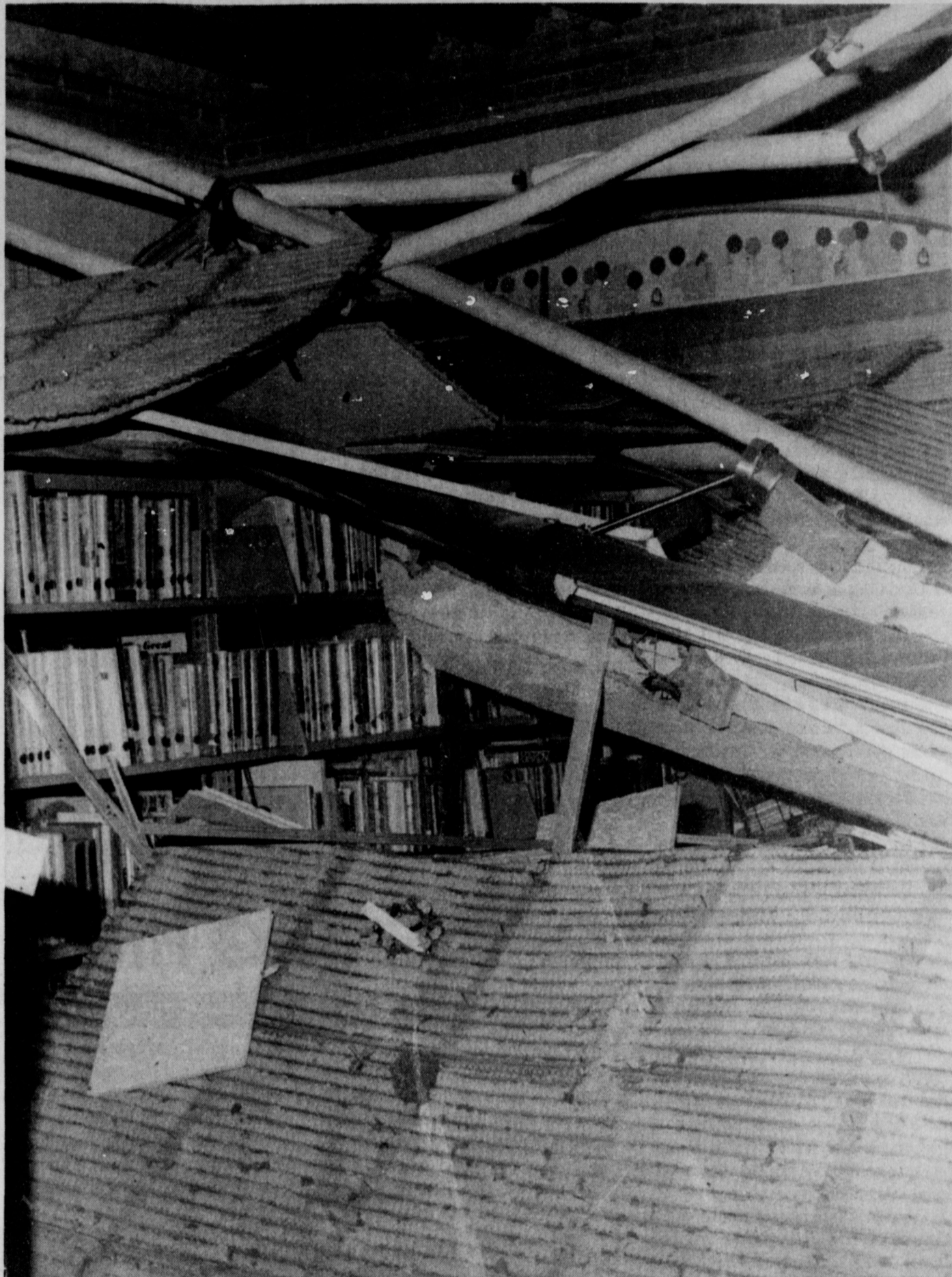
TREMENDOUS DAMAGE , though the amount is yet unknown, was inflicted on the children's department of the Tom Burnett Memorial Library Saturday afternoon, when water caused the ceiling to cave in. Members of a wedding reception in the upstairs floor called police at 2:56 p.m. to report a loud noise. Upon investigation, it was determined a water leak had caused the heavy plaster ceiling to collapse into the room's interior. Authorities have been working through the week to determine the extent of damage to the structure, furniture and books. Most of the repairs are covered by insurance, but when they will be accomplished is yet to be determined.
