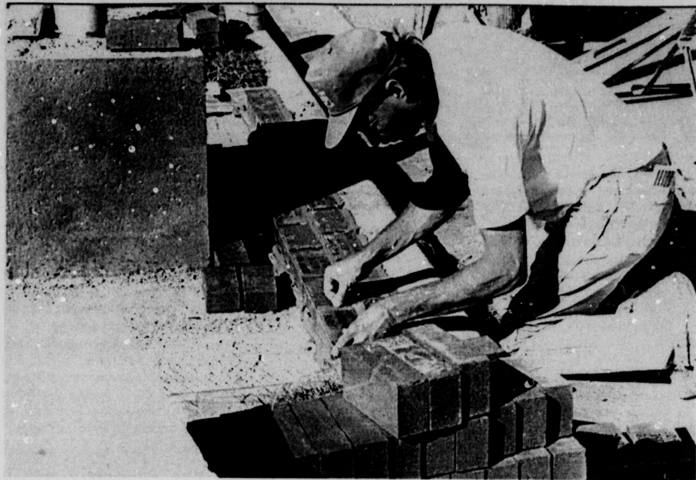
PERSONALIZED BRICKS now adorn the base of the newly-installed flag pole at the Recreational Activities Center. The bricks are an on-going fund-raising project of the Clean and Green Committee, with the money used to beautify the community. The bricks were laid this week by Bill (shown here) and Joe Hrcirik, after the flag pole was installed by Belvin Lytle and Billy Gilmore. Orders for personalized bricks will continue to be taken, and workers will be accepting them all day Saturday in front of the Iowa Park Leader office.
