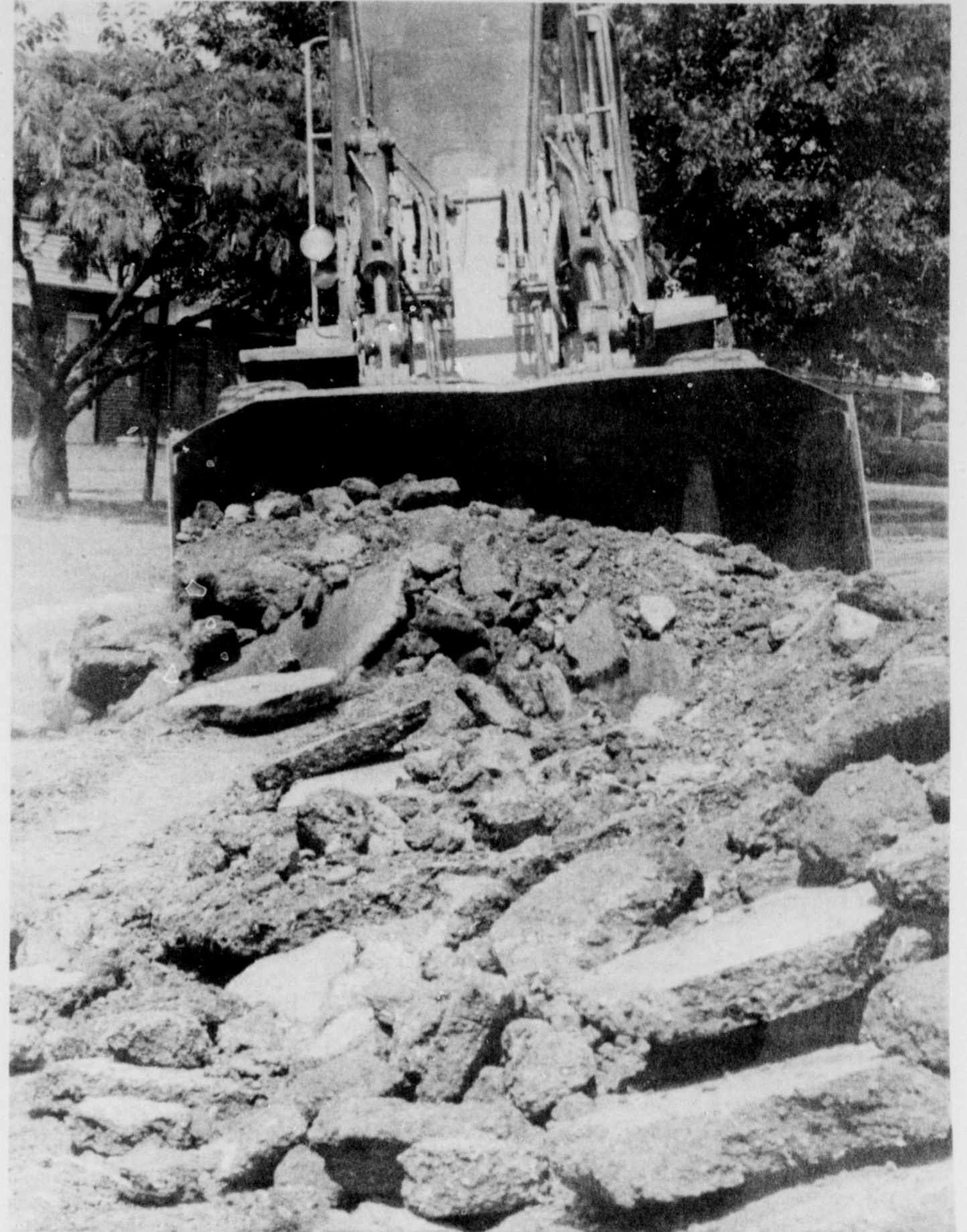
WELL ON THE WAY - Workers of the city's street department began this week clearing out the old pavement on Douglas so it can be resurfaced. The pavement was destroyed when a long-needed underground storm drain was installed at the intersection of Mary Drive, to carry the water to the Access Road. Work completion is expected within the next few weeks.
