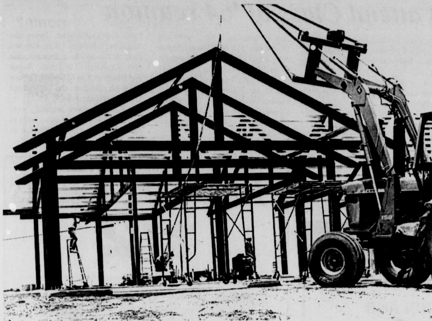
FIRST OF ITS KIND IN IOWA PARK is this steel-framed home under construction at 512 W. Coleman. It is being built by Park Builders, a newly-formed local corporation.
