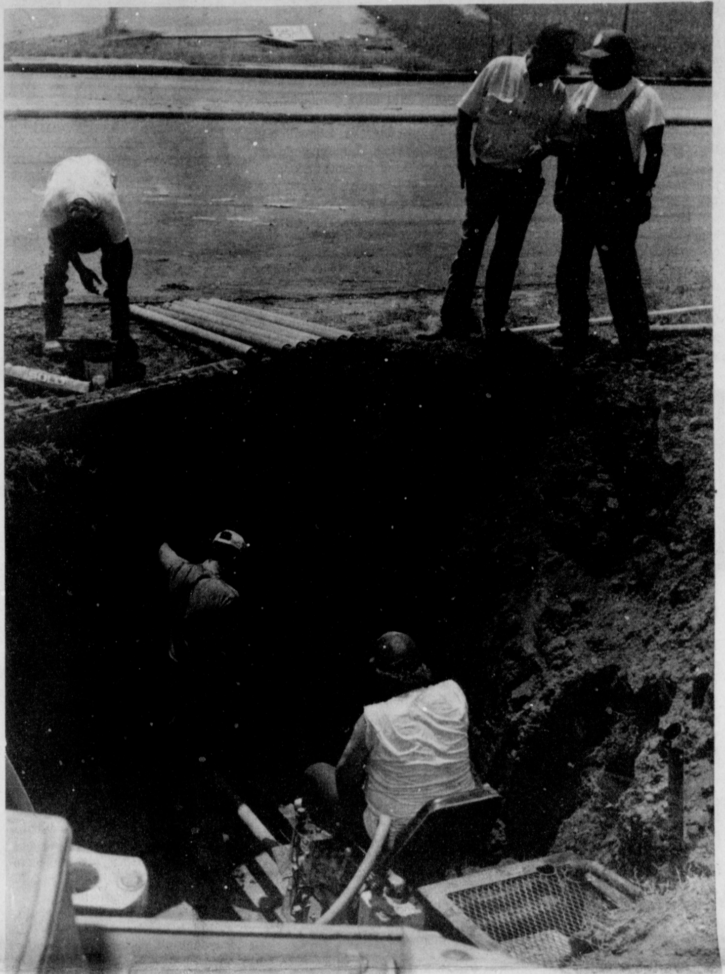
BORING WORK - Bowles Construction workers are shown making their final boring of the Westbound Access Road for a water line that will be connected with the new water tower just West of Johnson Road. They didn't have as much problem with this phase as they did when attempting to bore Johnson Road, where they found numerous water and natural gas lines that were not on any of the maps, delaying their progress by more than a week.
