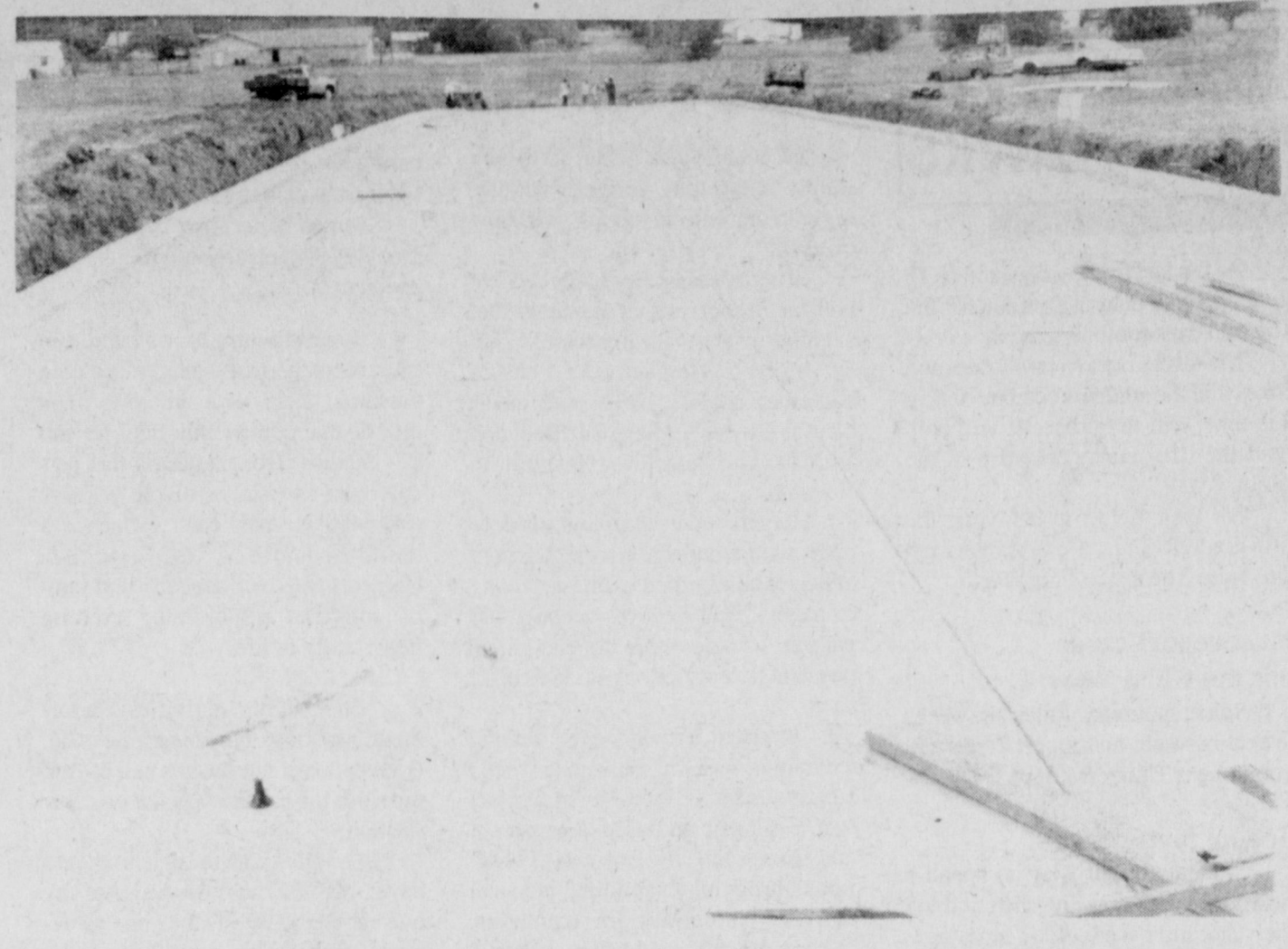
IOWA PARK'S NEWEST STREET, the 700 block of Aldine, is almost complete and ready for the city's newest housing addition.
