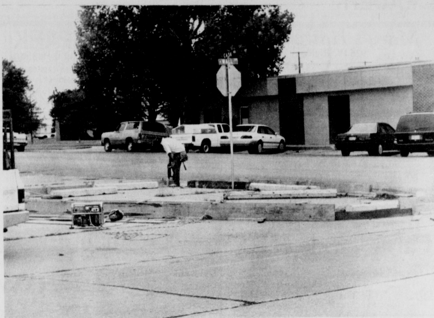
A PLACE OF FUTURE BEAUTY - The northeast corner of Wall and Cash is undergoing work that will transform it into a place of beauty in the future. Workmen are laying a concrete curb away from the sidewalk, and removing the concrete pavement, for a mini park site. It's all part of the community's beautification effort.
