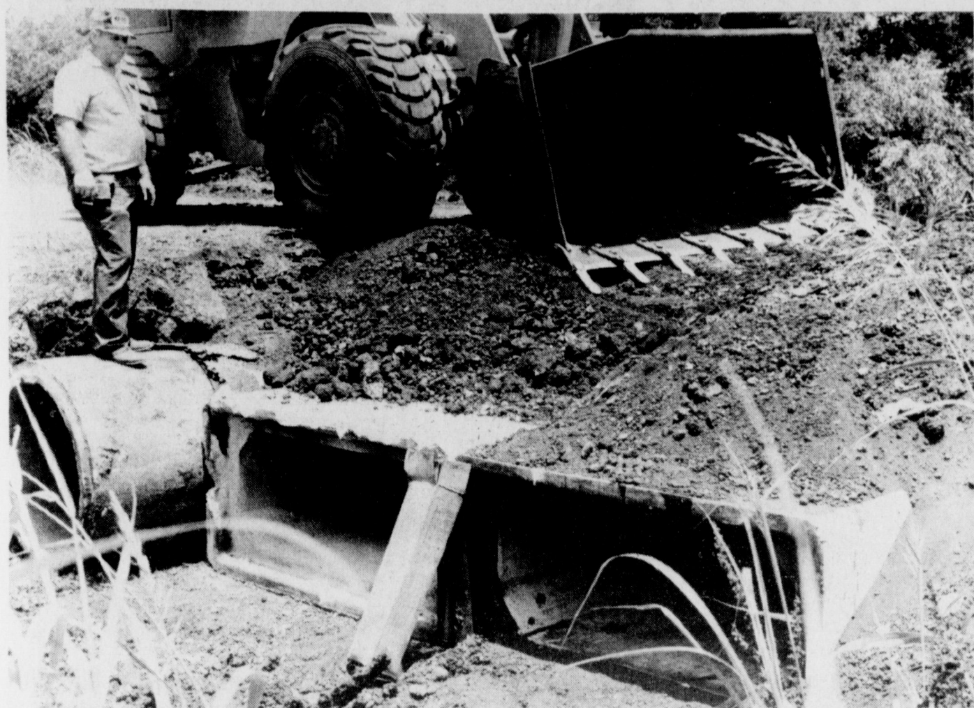
BIGGER AND BETTER - A new bridge was put in place on Bell Road Wednesday of last week, by County Commissioner Gordon Griffith and his crew. The larger concrete culverts are expected to allow water to flow faster, and the crossing is considerably wider than the original. A similar crossing is planned for North Victoria this fall.
