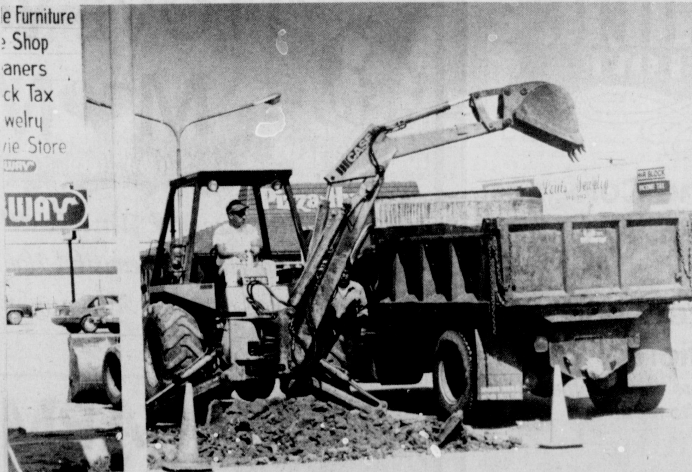
WORK BEGAN this week to open the 400 block of West Park through Park West Shopping Center. The first phase of the project will be construction of curb and gutters.
