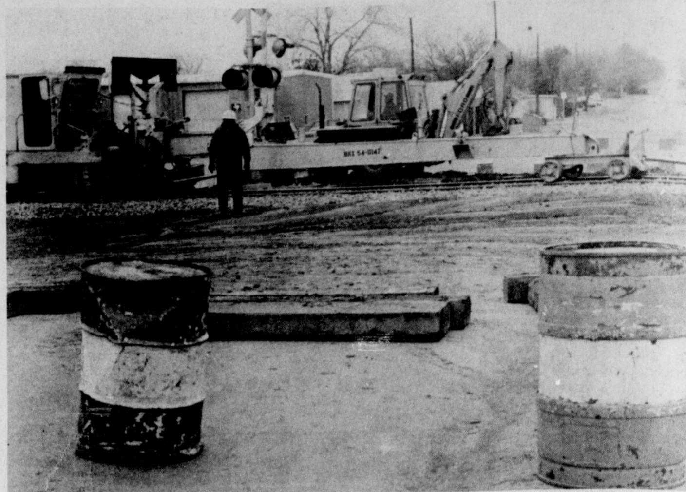
CROSSING IMPROVEMENTS - A crew from Burlington Northern Railroad has been working almost two weeks, removing the old, standard wooden cross-ties and replacing them with either concrete or rubber ties. Concrete was used at the Wall and Jackson crossings. The rubber ties are expected to be used on the Yosemite crossing.
