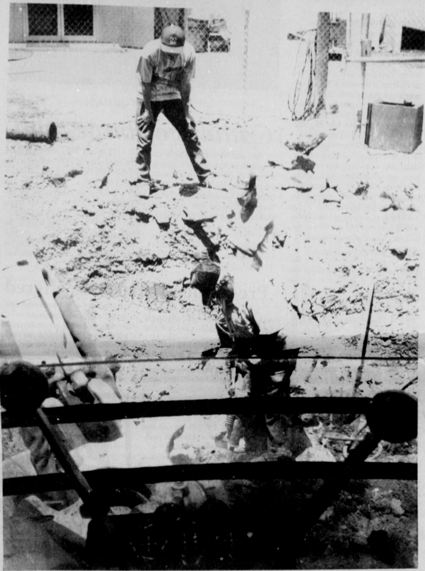
DIGGING OUT THE PROBLEM - Texas Street was closed this week in front of the city's water treatment plant, as workers dug out a large line where a leak had developed. The problem was first noticed when the surface beside the bulk water pump began crumbling. Early attempts to shore up the problem with concrete failed, when it was determined the soil was saturated.
