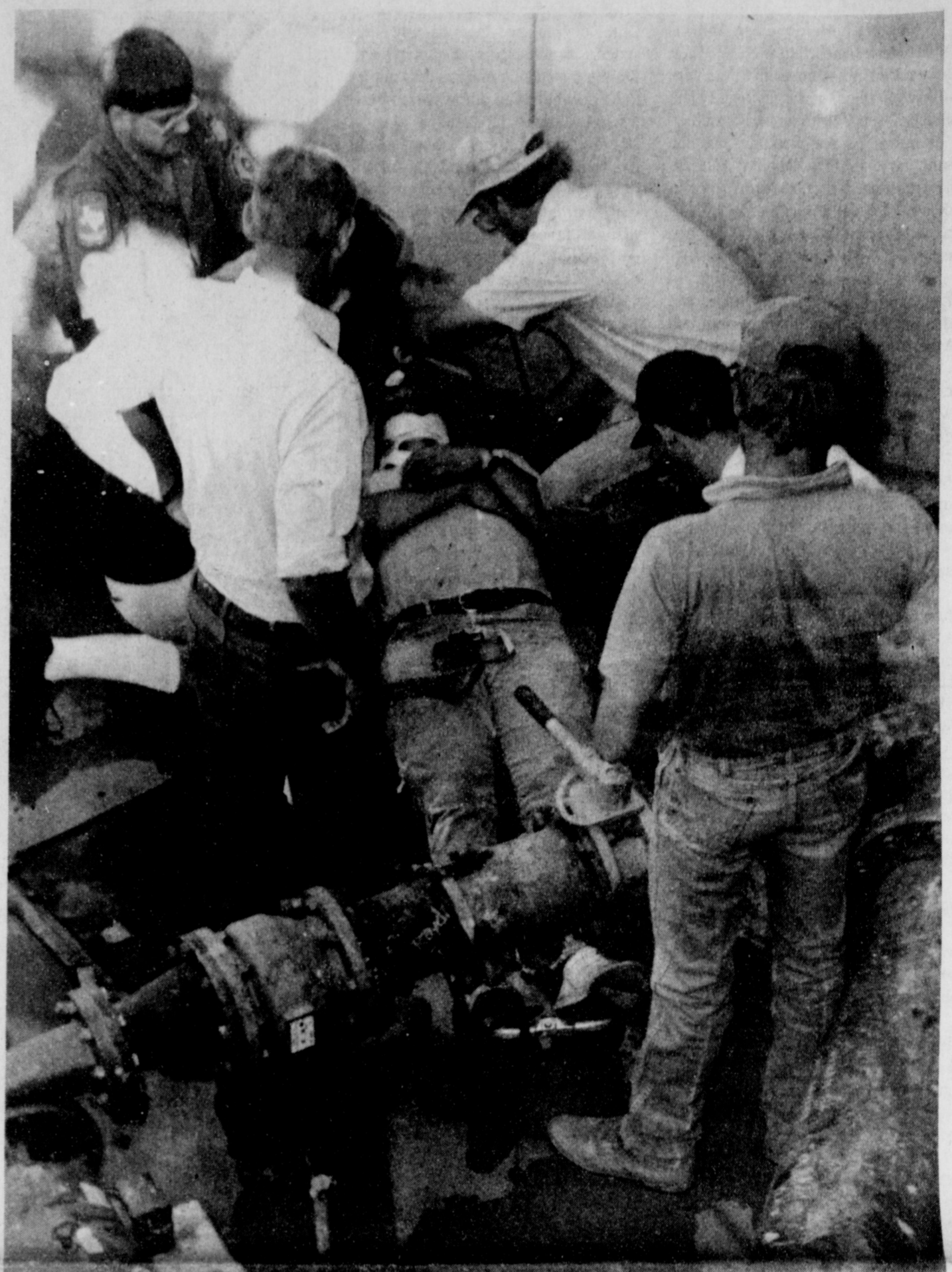
SURVIVES LONG FALL - Iowa Park EMTs prepare Bradford Boyd to be lifted out of a 14-foot-deep concrete pit after he fell some 26 feet Tuesday afternoon. Boyd, an employee of a contractor building a transfer pump station at the city's water treatment plant, was taken by ambulance to a Wichita Falls hospital, where he was treated for a minor head wound and released. He had been working on the building's framework at the time of the accident.
