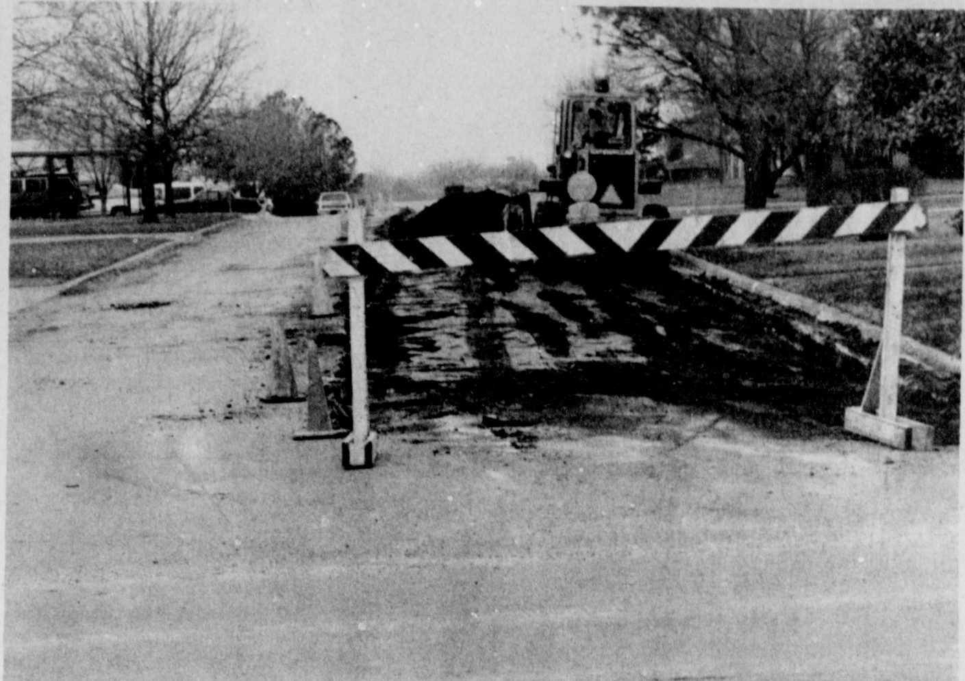
PROJECT UNDERWAY - City employees began the process Monday of rebuilding the 500 block of West Clara. Half the street's width will be worked at a time, to allow passage. Materials from the street will be used in alleys. The project is a part of the city's aggressive street improvement program.
