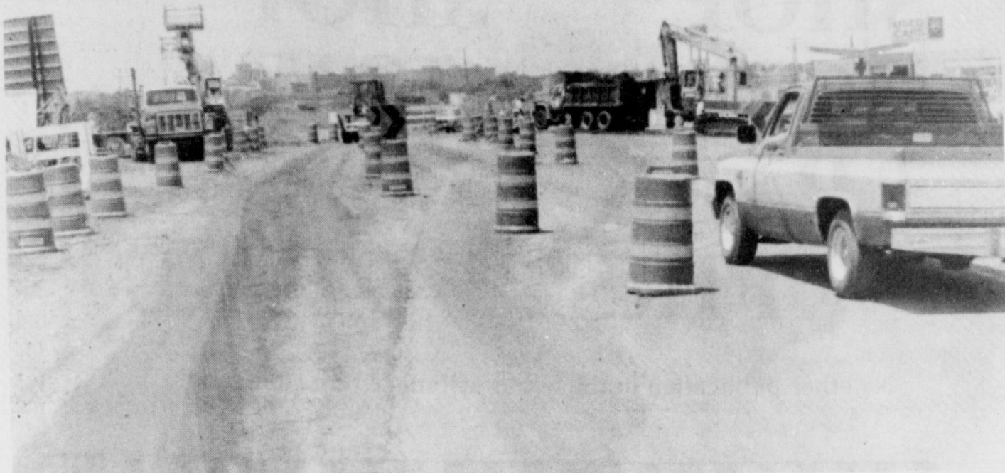
DETOUR ON WEST HIGHWAY - Construction workers had to detour traffic at two different locations this week on West Highway, to lay new concrete culverts, in preparation for widening the thoroughfare into three lanes.
