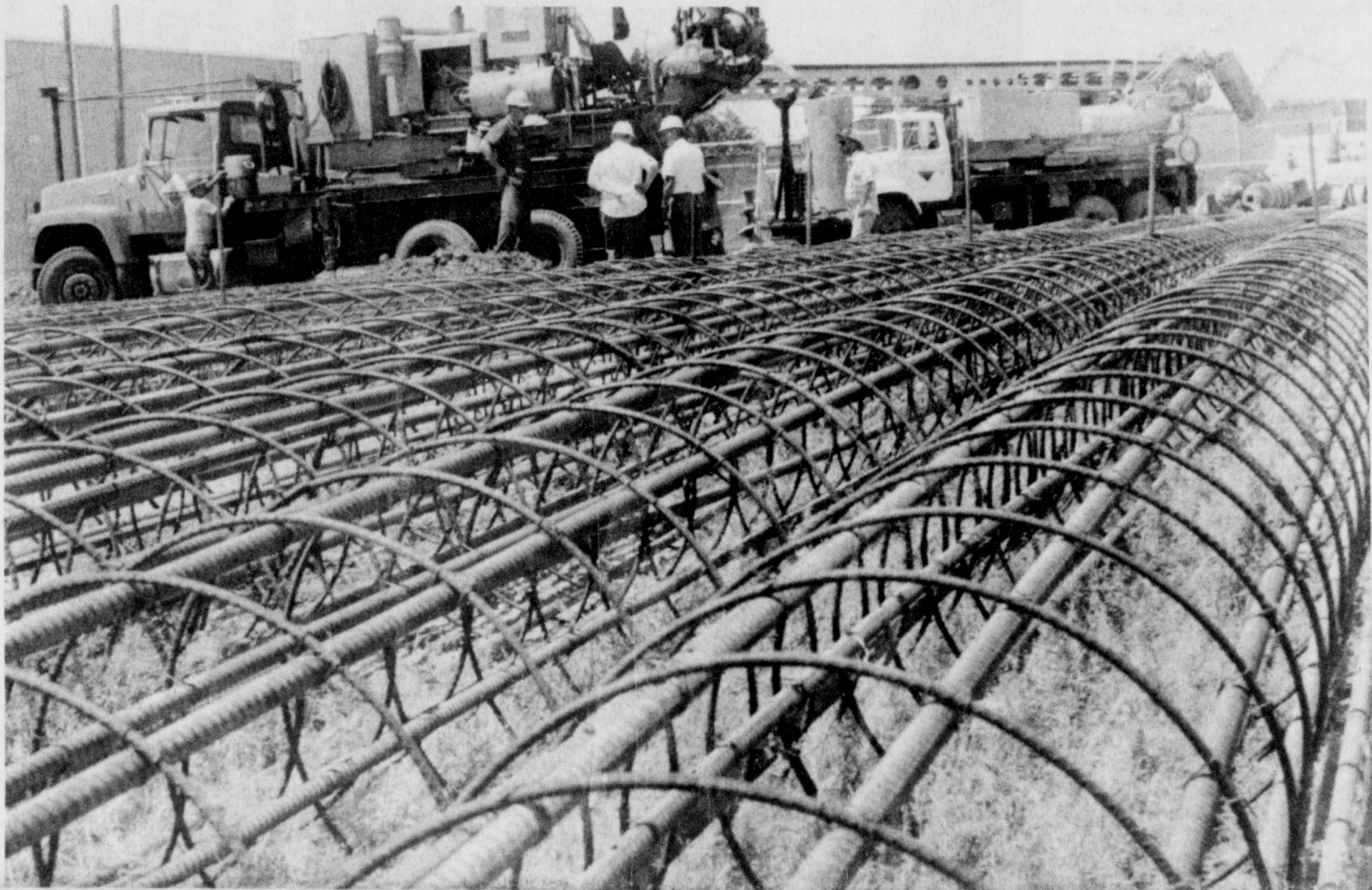
A MAJOR ADDITION to Iowa Park Junior High School is underway, as workers this week drilled pier holes to support the nine-classroom wing. Steel for
