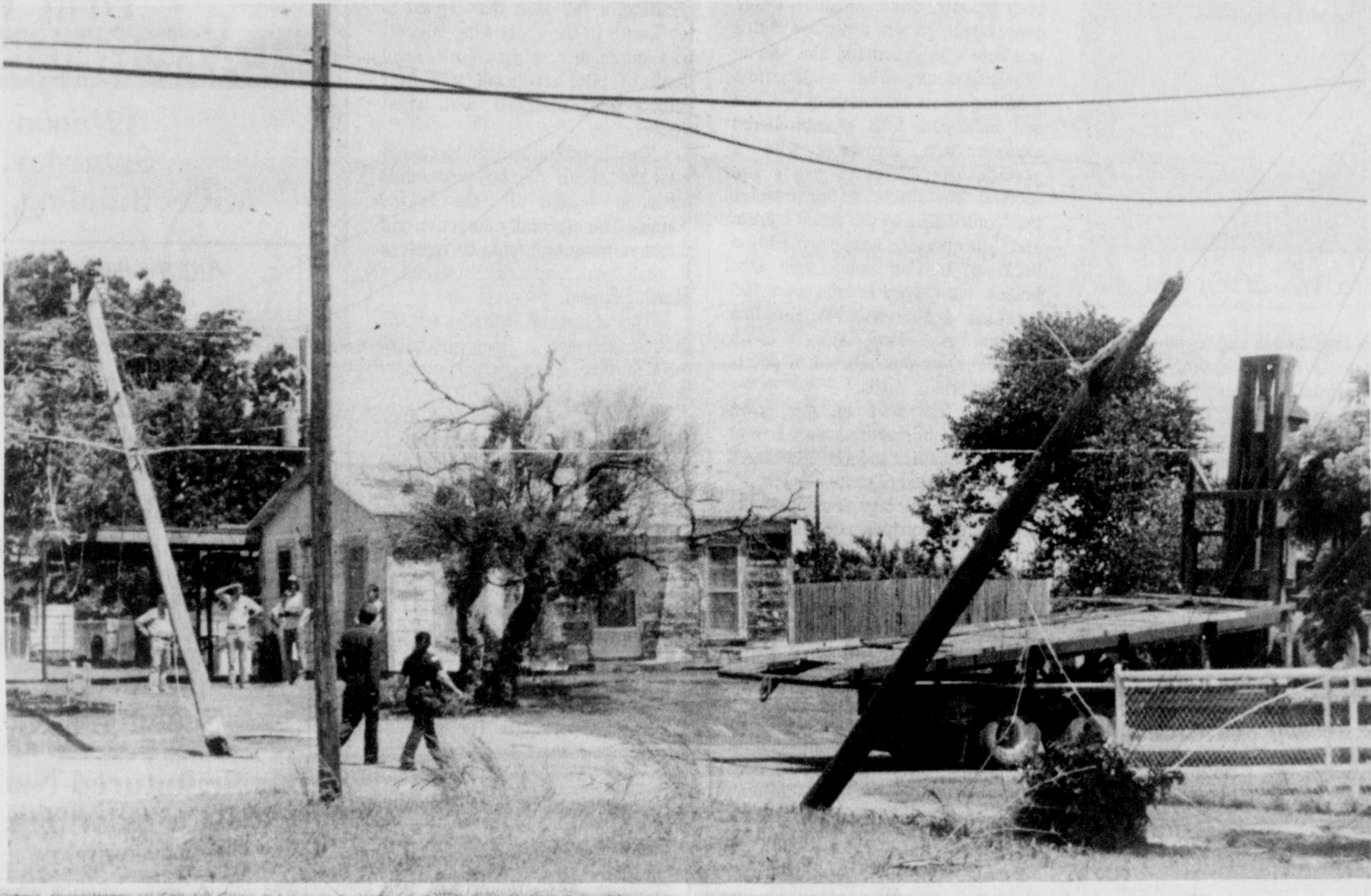
UTILITY SERVICE was disrupted to much of the southern portion of Iowa Park Friday afternoon, when a Barbour Trucking driver failed to lower a forklift unit and snagged overhead lines in the 600 block of
