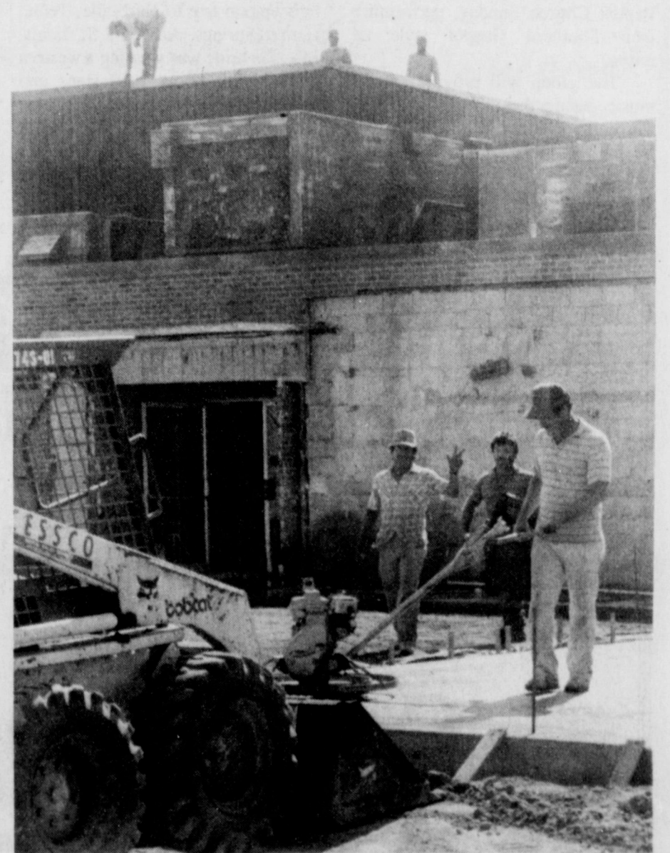
WORK on the high school expansion and remodeling project is well underway this week, as the floor of the music department is poured and replacement of the 20-year-old roof is about to start.
