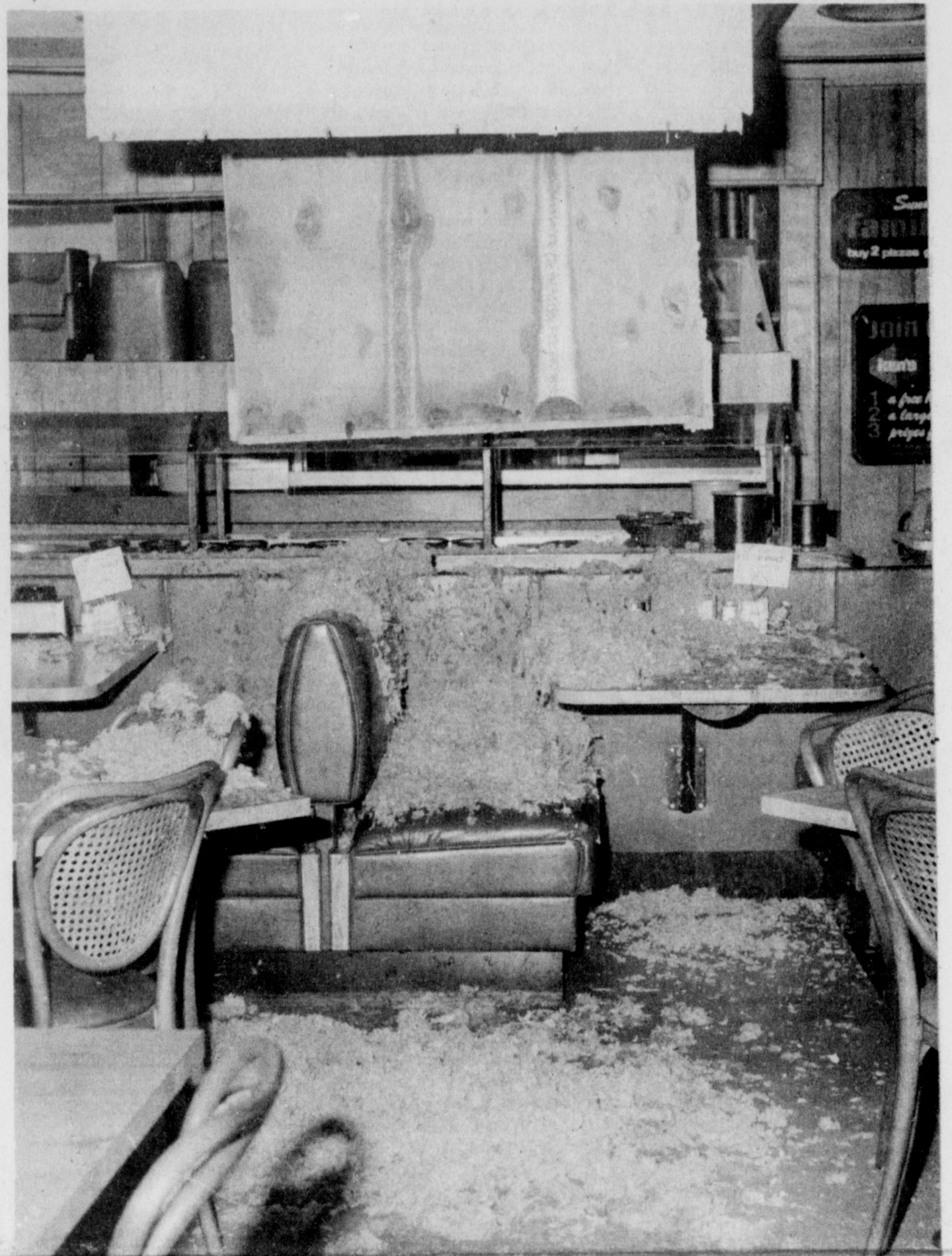
INTERIOR OF KEN'S PIZZA TUESDAY MORNING ... after storm damaged roof and ceiling collapsed.
