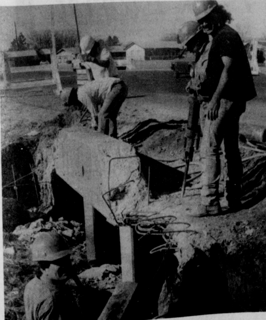
WORKERS BEGAN preparation work this week for the widening of West Highway between Colorado and Johnson Road. When completed, a third lane will be available for left turns only.
