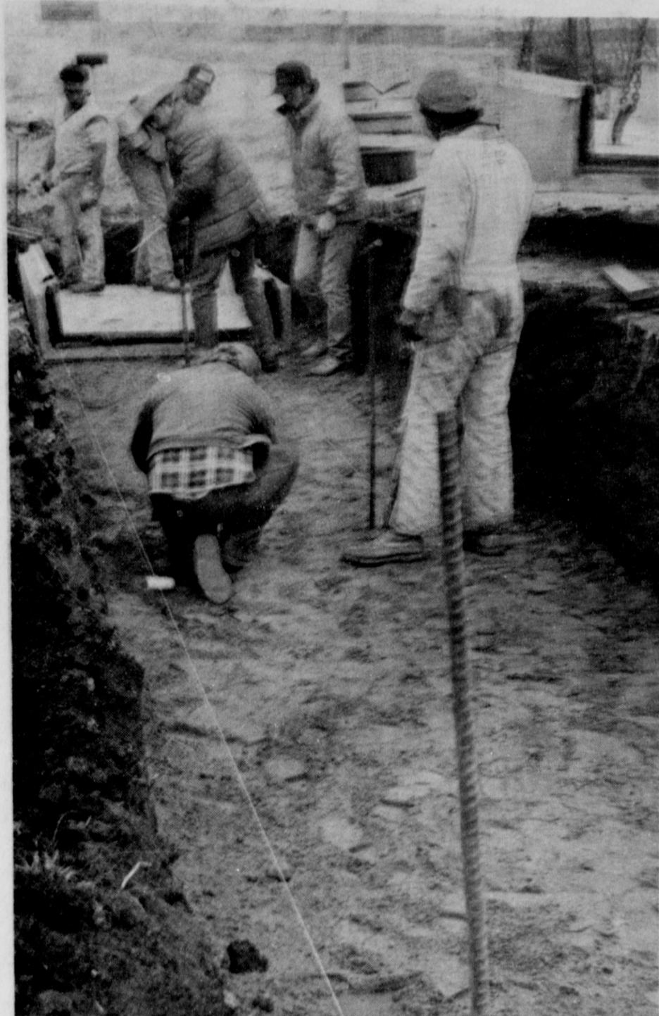
FIRST CULVERT of two planned for South Wall was put into place Tuesday by construction workers. The street is to be widened and completely rebuilt from the railroad tracks to Garden Valley.
