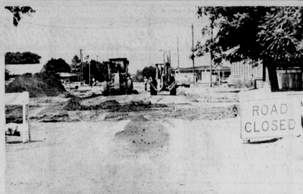
WORKERS PREPARE the 100 block of South Victoria for a new concrete surface. The project is part of an overall city program to replace old asphalt paving.
