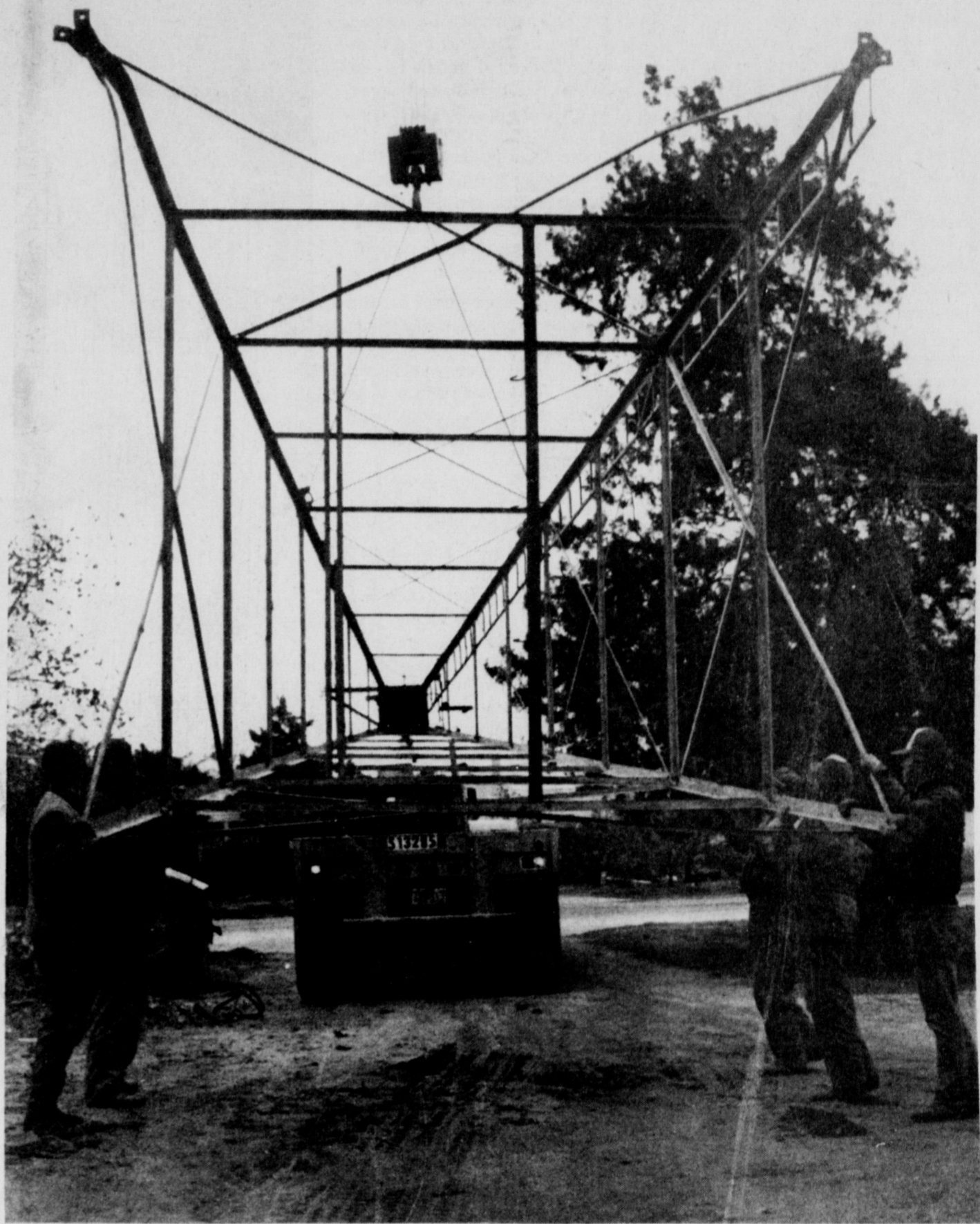
SKYLINE LANDMARK REMOVED - Workmen took down the old metal tower which has stood decades behind the city hall. The fire siren it had held was moved to the water tower. The metal structure has been relocated by the fire department's south station, where it will hold antennas and another siren, and will benefit the fire and police departments' emergency backup radio.
