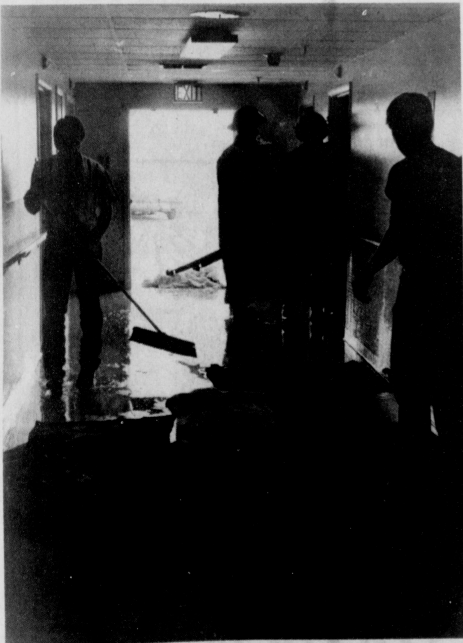
MESSY AFTERMATH - While firemen were relieved Sunday that the alarm at Heritage Manor was not a fire, employees weren't too happy with the mess that caused the fuss. Pipes in the ceiling carrying water to the sprinkler system froze and burst, flooding much of the north wing of the building.
