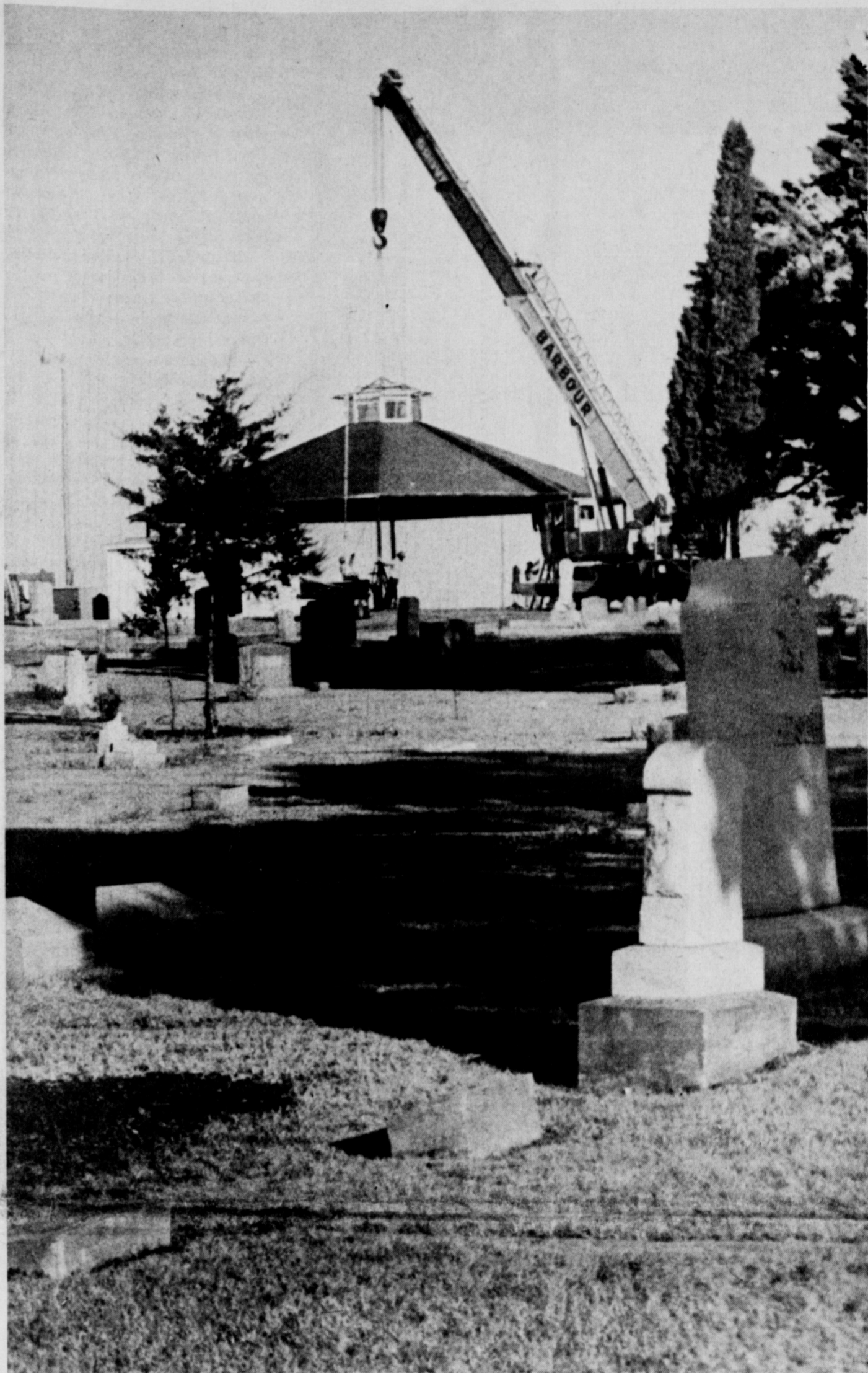
CEMETERY PAVILLION - Workers of Gilmore Inc. and Barbour Trucking put the pre-built roof Tuesday on the new pavilion under construction at Highland Cemetery. The structure will feature an open air area where gatherings and services can be held, as well as an office, rest room and storage area. Construction is being financed primarily by volunteer donations.
