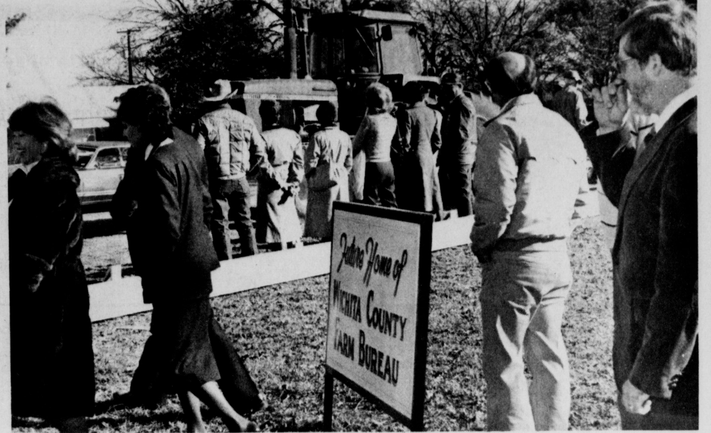
UNIQUE GROUNDBREAKING - Wichita County Farm Bureau president Fred Dwyer plowed a strip of land as workmen put up foundation forms for the organization's new office across the street from the post office, while dozens of members and well-wishers looked on. The event took place Monday morning.
