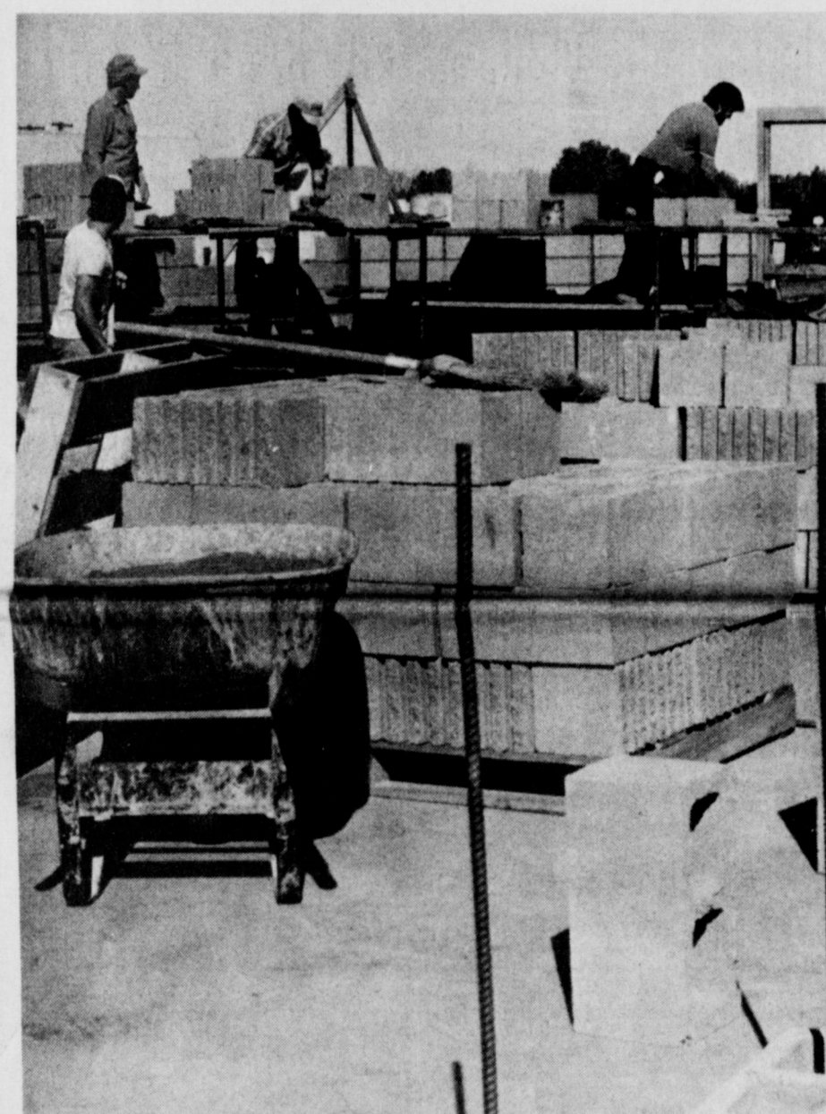
WALLS GOING UP ON NEW EATING BUSINESS ... at a corner of West Highway and Pacific.
