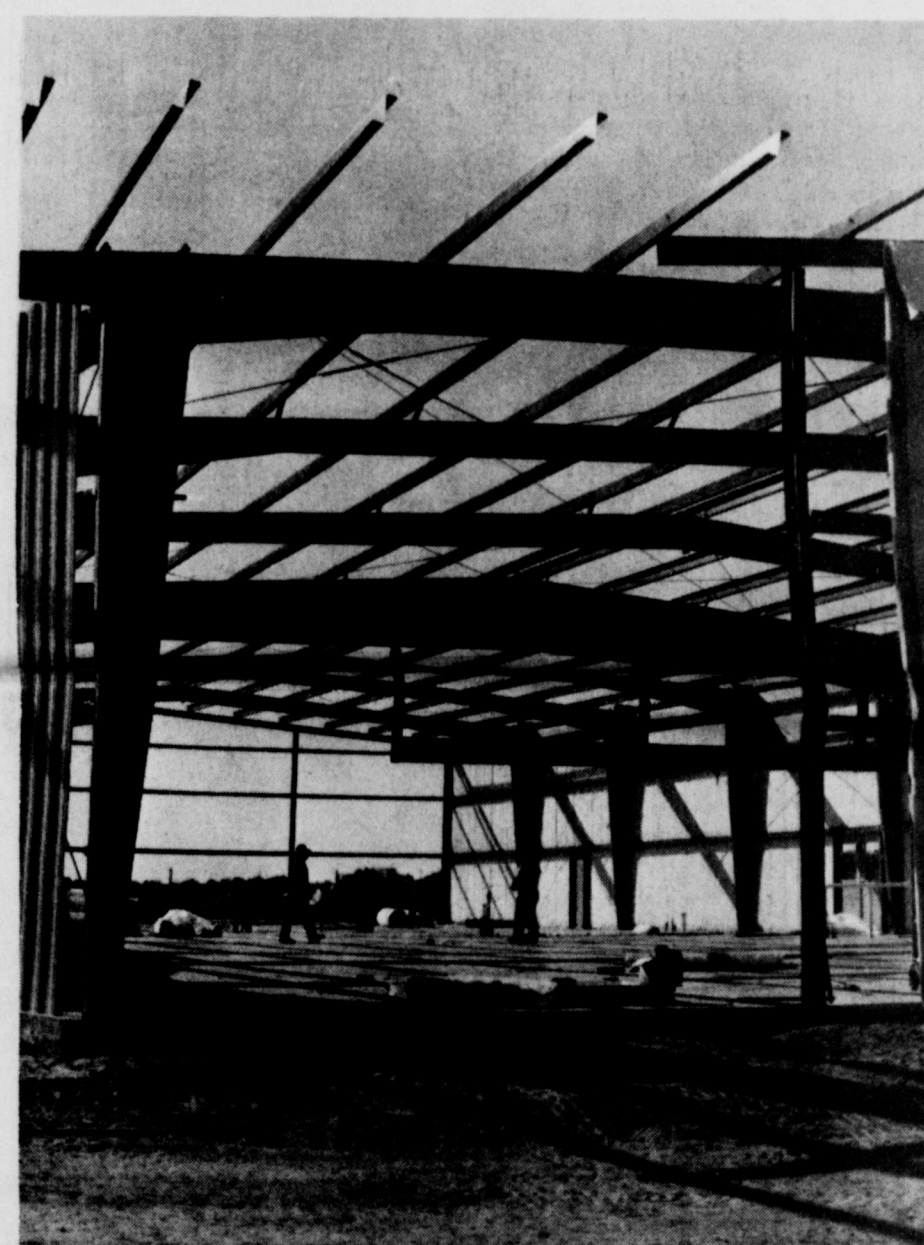
ABOUT READY FOR ROOF OF NEW CHURCH BUILDING ...for Lakeview Church of God.
