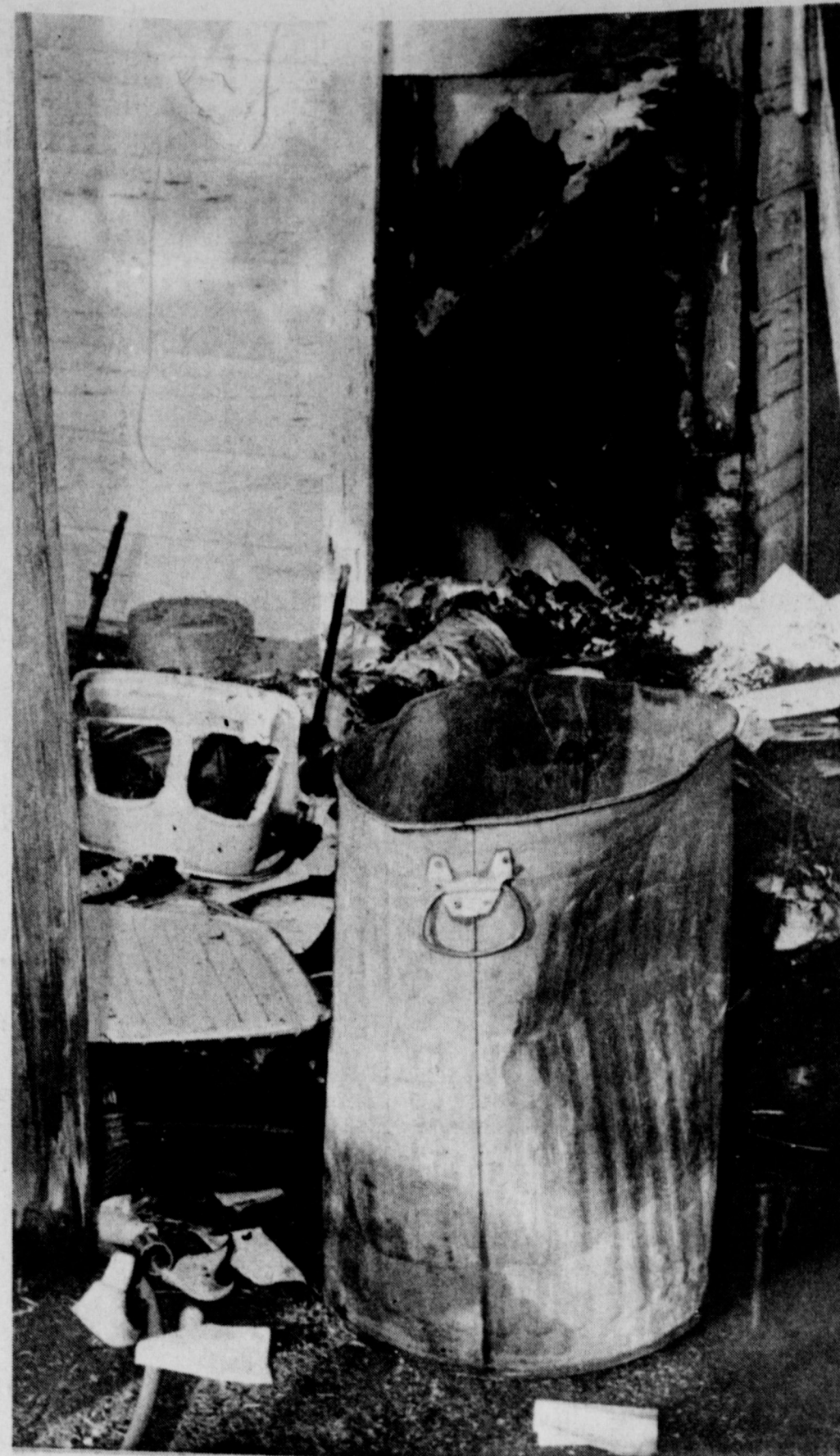
HOT TRASH - Trash in this metal can caught fire while sitting next to the house at 415 W. Daisy Tuesday afternoon, igniting the wooden walls. Firemen extinguished the blaze before major damage was done to the structure.
