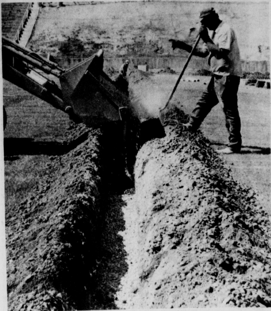
DRAINAGE PROJECT UNDERWAY - Workmen began this week with an underground drainage project at Hawk Stadium, designed to carry away high-level salt water that threatens to kill turf on the field. The project is expected to be completed by mid August.
