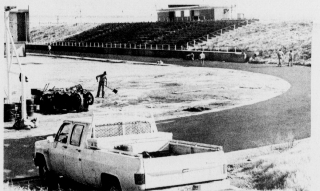
WORKMEN took advantage of good weather conditions Tuesday to complete much of the work of rebuilding and resurfacing the track in Hawk Stadium.
