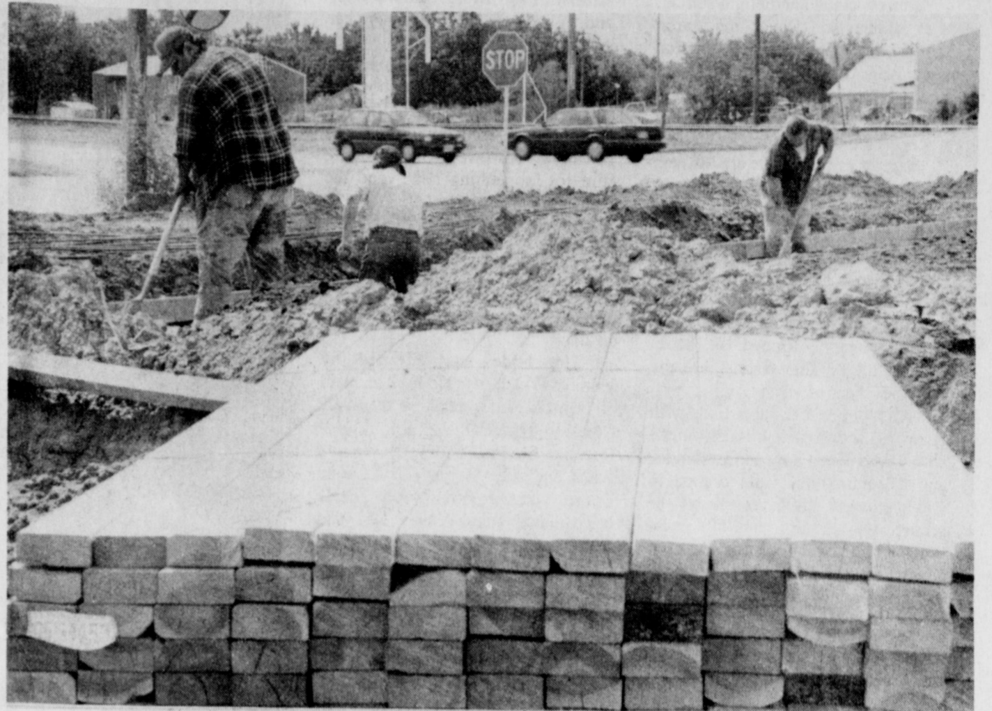
WORK UNDERWAY - With installation of plumbing and preparations completed for foundation and floor pouring, the new Chamber of Commerce office is about to begin taking shape. It will be located at the northwest corner of East Highway and Wall.
