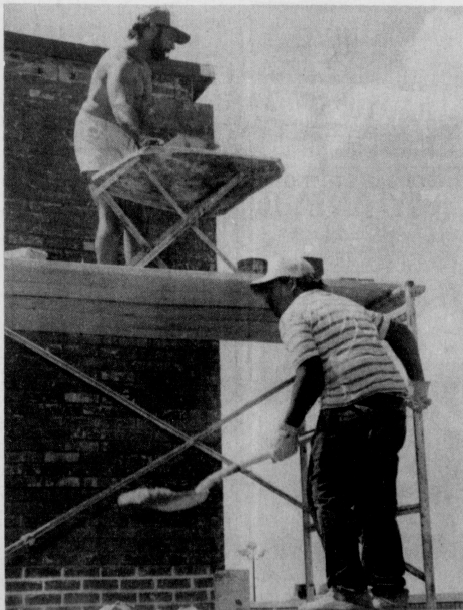
BRICK LAYING in 100-degree temperatures and no shade is a hard life, but somebody's gotta do it. These two workers were busy completing a repair project on the high school gymnasium.
