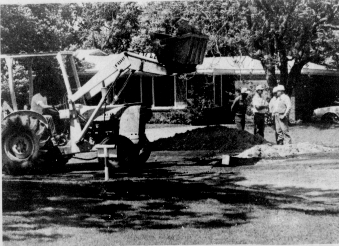
CLEANING UP MESS - Texaco workers had a mess on their hands with an eight-inch oil transmission line ruptured at the intersection of Jefferson and Yosemite Monday. It was reported to police at 4:30 p.m. A clamp corrected the problem and temporary repairs on Yosemite were made Tuesday. The line was installed in 1920, according to one of the workers.
