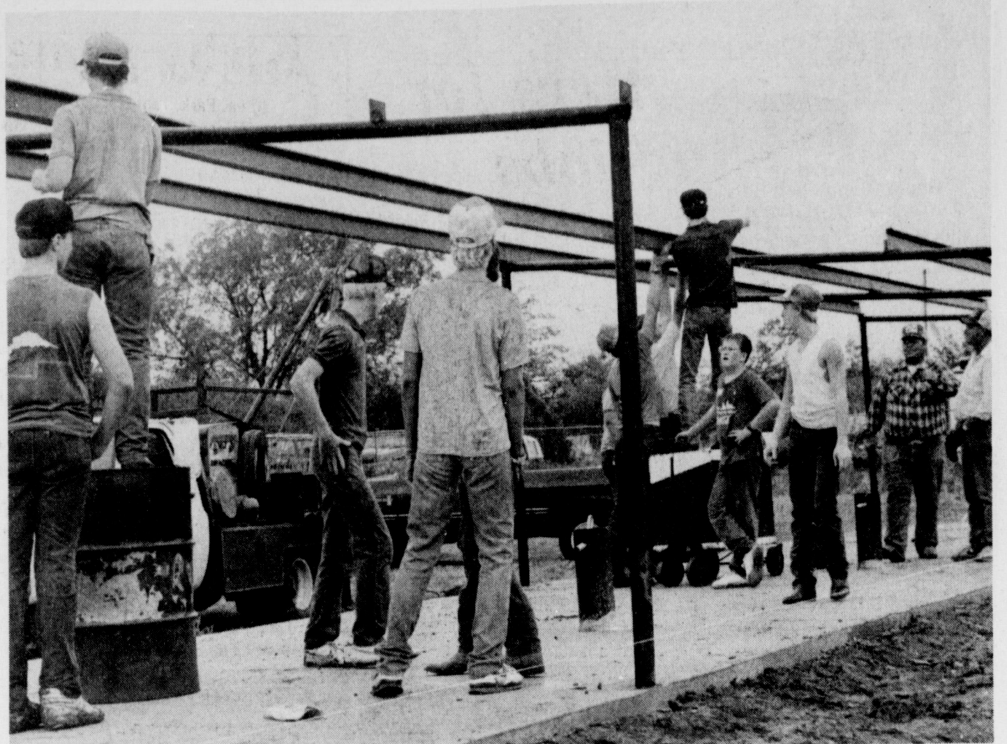
GOING UP - Members of the high school's Vocational Agriculture department, with the assistance of Wichita County Young Farmers and FFA Booster Club members, are building new sheds at the Ag Farm in the southeast part of town. Their work Saturday morning finally came to an end, however, when the rains began falling steadily.
