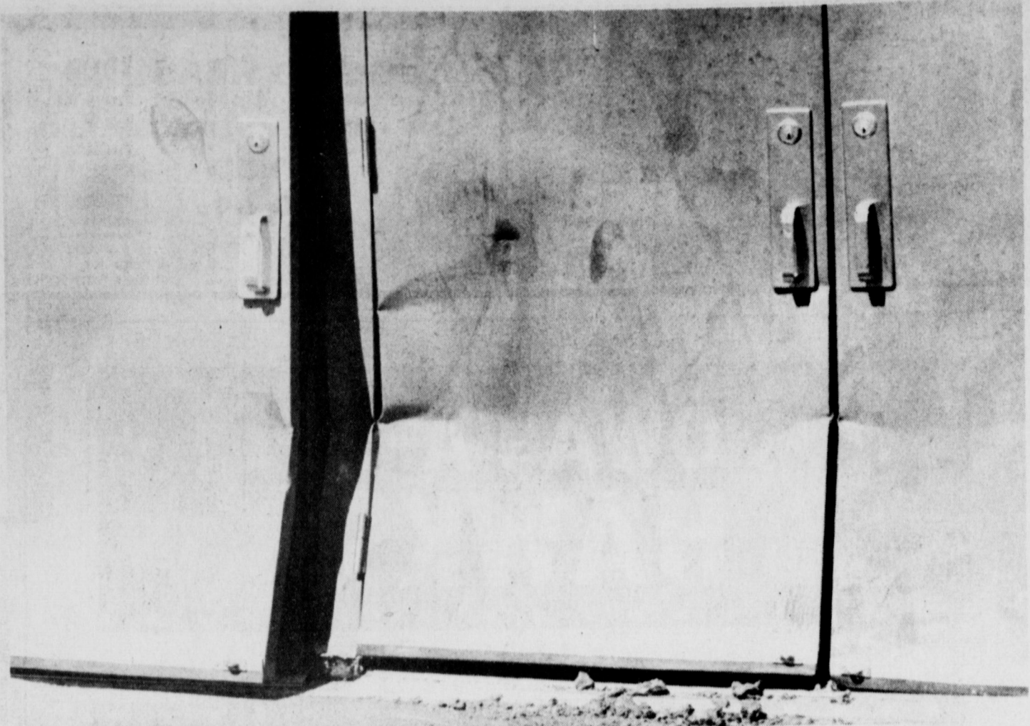
EXPENSIVE VANDALISM - Someone caused several thousand dollars worth of damage the weekend of Sept. 8-9 to the triple-door entrance on the east end of the new high school gymnasium. Officials say a dual-wheeled truck, possibly with a welding bed, destroyed the doors and
