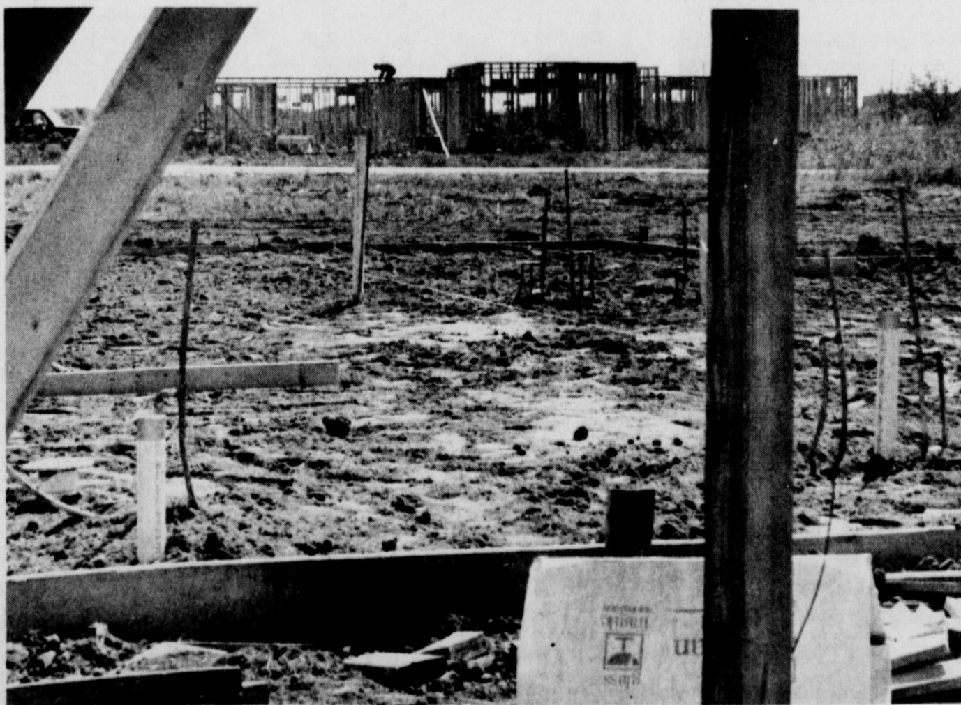
HOME CONSTRUCTION is booming in the Quail Valley area, where four new residences are presently under construction and land has been cleared in preparation for
