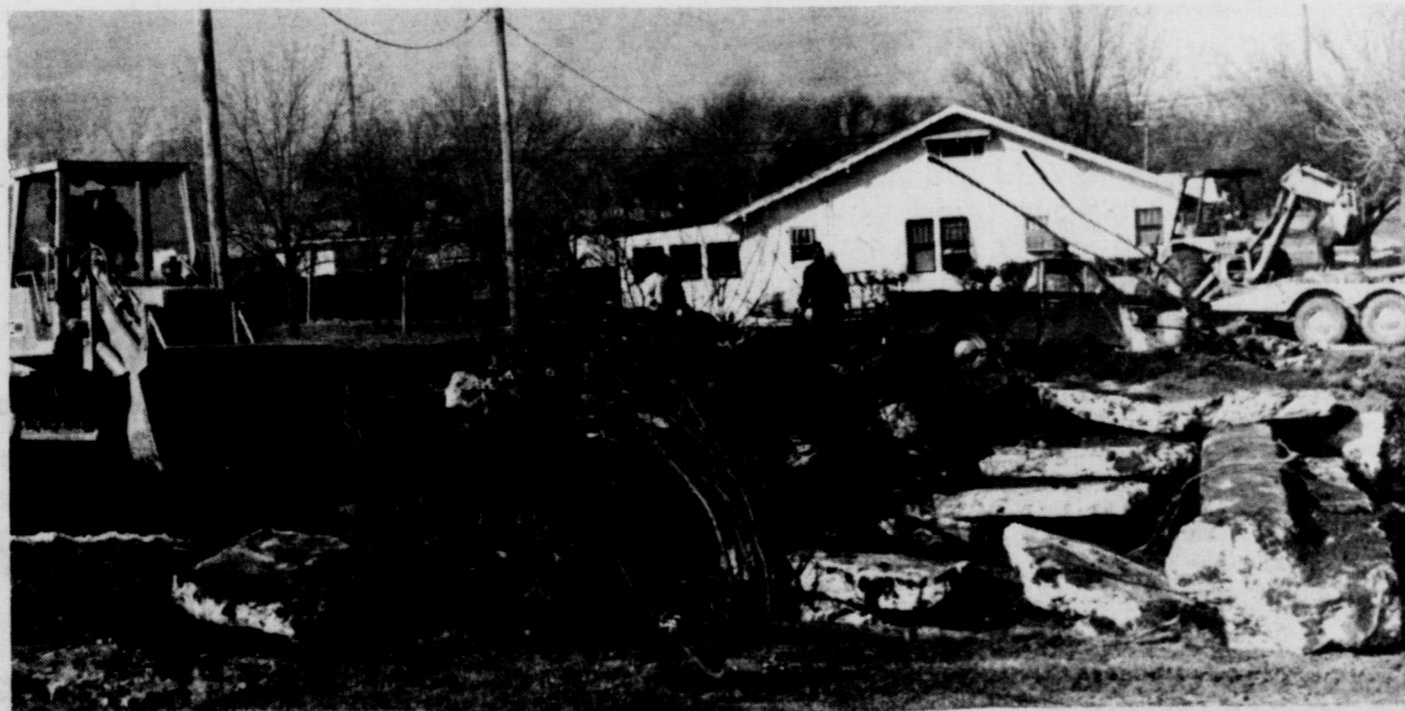
LOT CLEARED - The old "Brubaker Building" site at Bank and Wall was cleared this week. State National Bank plans to pave it for employee parking sometime in the future.
