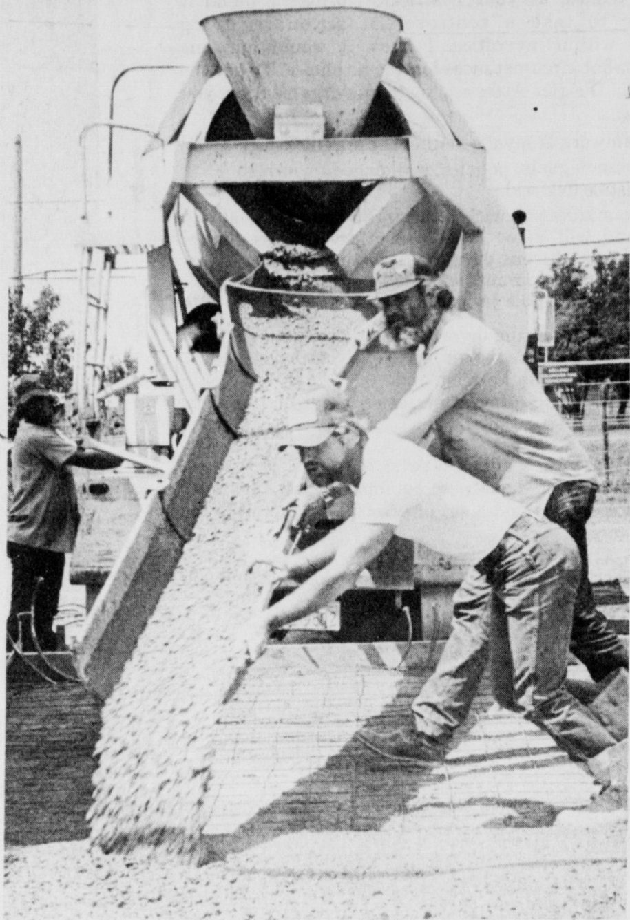
NEW ADDITION for the Holliday Volunteer Fire Department got off the ground Tuesday with volunteers pouring concrete for the slab. The addition, which will house the future offices of the Archer County Sheriff's Department and Department of Public Safety, but will also have a municipal courtroom and office space for what city officials hope is a future fulltime justice of the peace.
