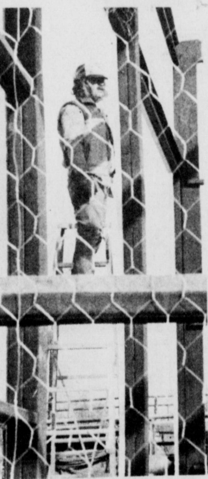
BUILDING PROGRESS - Workmen began Tuesday putting the metal siding and insulation on the Volunteer Fire Department sub-station on South Texowa. The exterior is expected to be completed by today.
