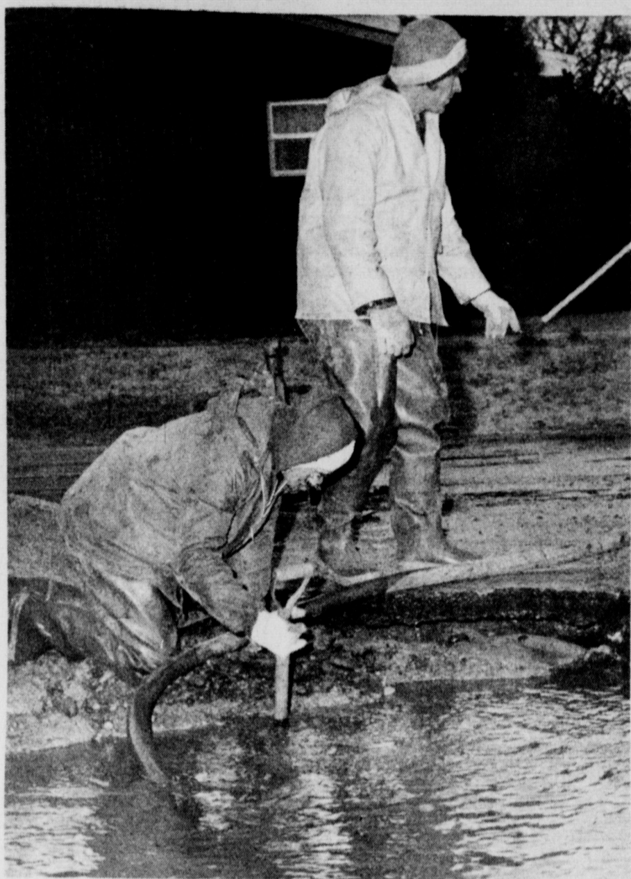
MAJOR LINE BREAK - The entire community's water system was shut down almost an hour and a half Friday afternoon when an eight-inch main broke at Wall and Aldine. Workmen had to drain the system in order to reach and repair the pipe.
