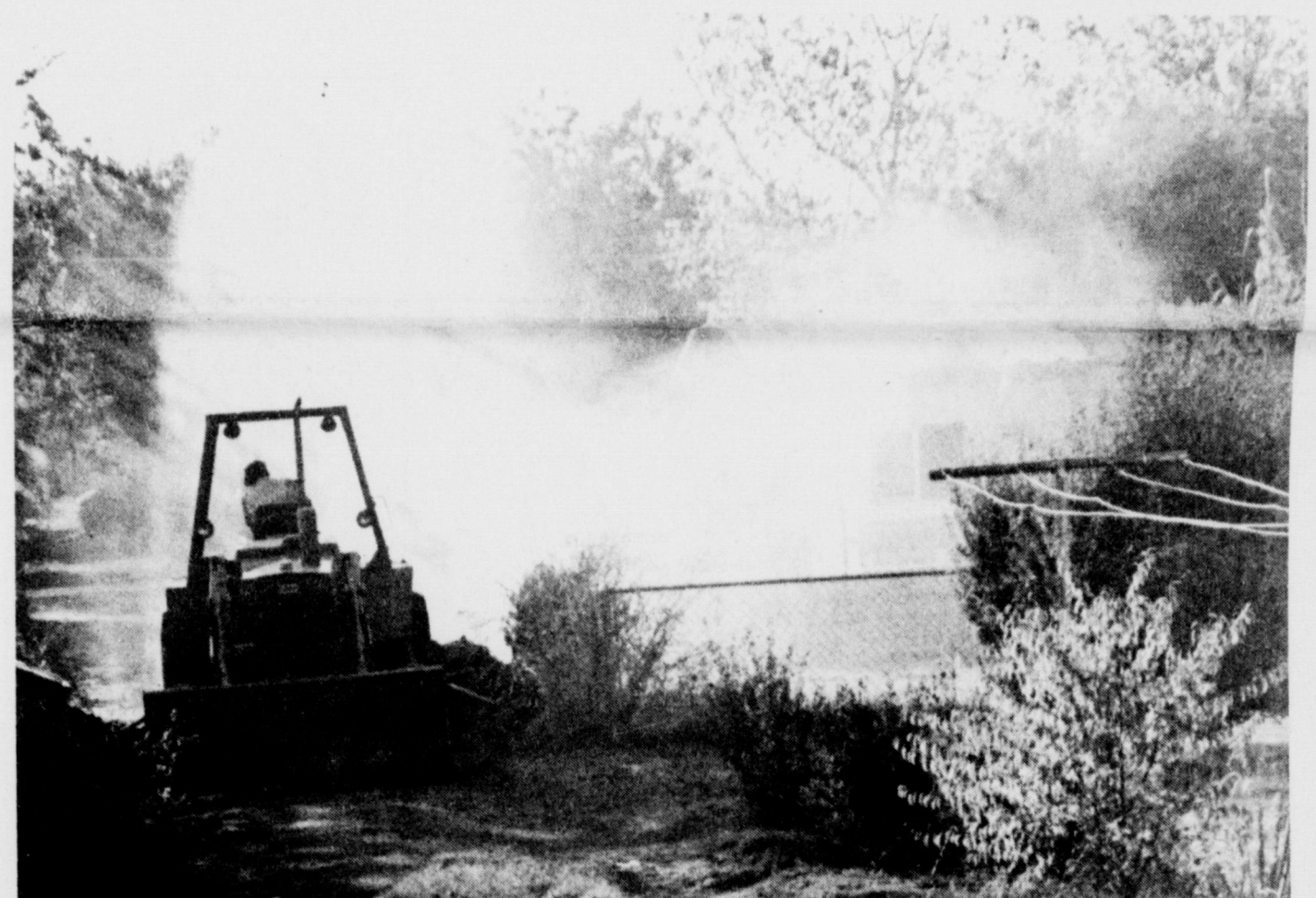
NATURAL GAS SPRAY - City workers late Wednesday of last week were digging to repair a water line leak when a Lone Star Gas pipeline was broken. Employees, at the direction of local utility manager Bud Burch continued digging to expose both lines so both could be sealed. The pressure of the natural gas combined with water from the
