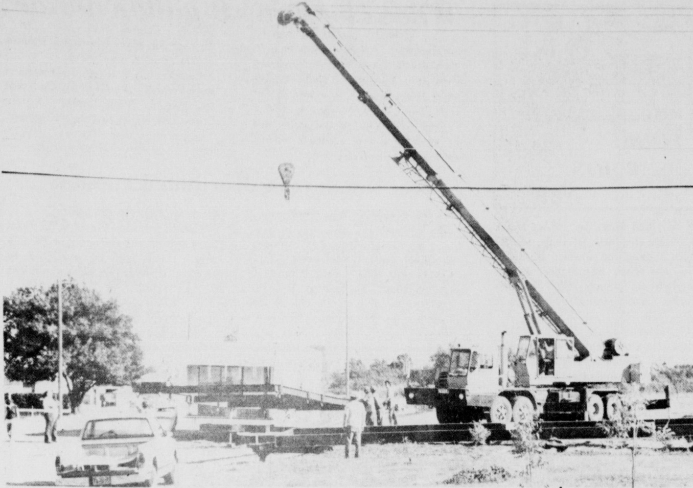
BUILDING BLOCK APARTMENTS - Prefabricated sections of a five-unit apartment complex were put into place Saturday afternoon on First Street, just north of the
