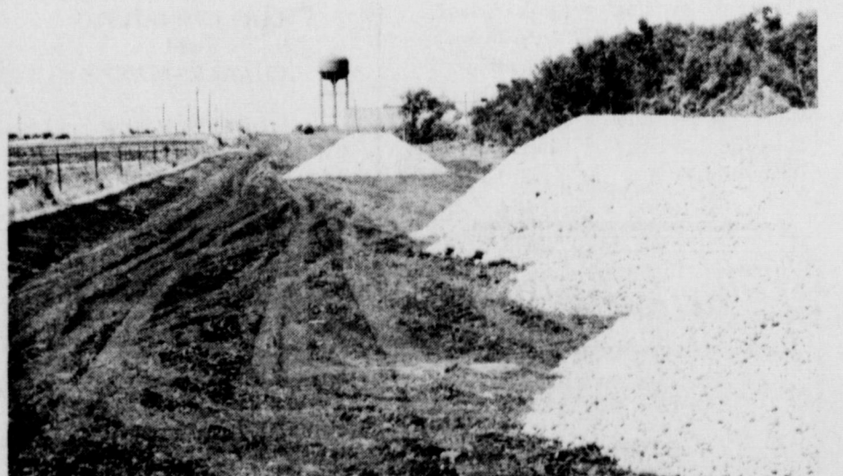
NEW LANDFILL ROAD - City crews are building an all-weather surface from Smith Road to the new sanitary landfill, southwest of the city. The entrance is slightly offset from Smith's intersection with Johnson Road. The new landfill is expected to be in operation by October.
