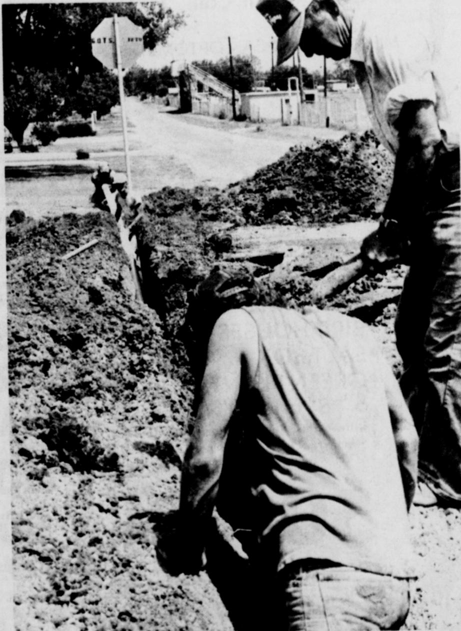
REPLACING LINE - An indication of why the city is hoping for a $100,000 matching grant from the federal government to replace old water lines was made evident this week. After patching a line at Bank and Victoria three times recently, workers finally had to dig across the pavement to lay a new section of line that couldn't be patched again.
