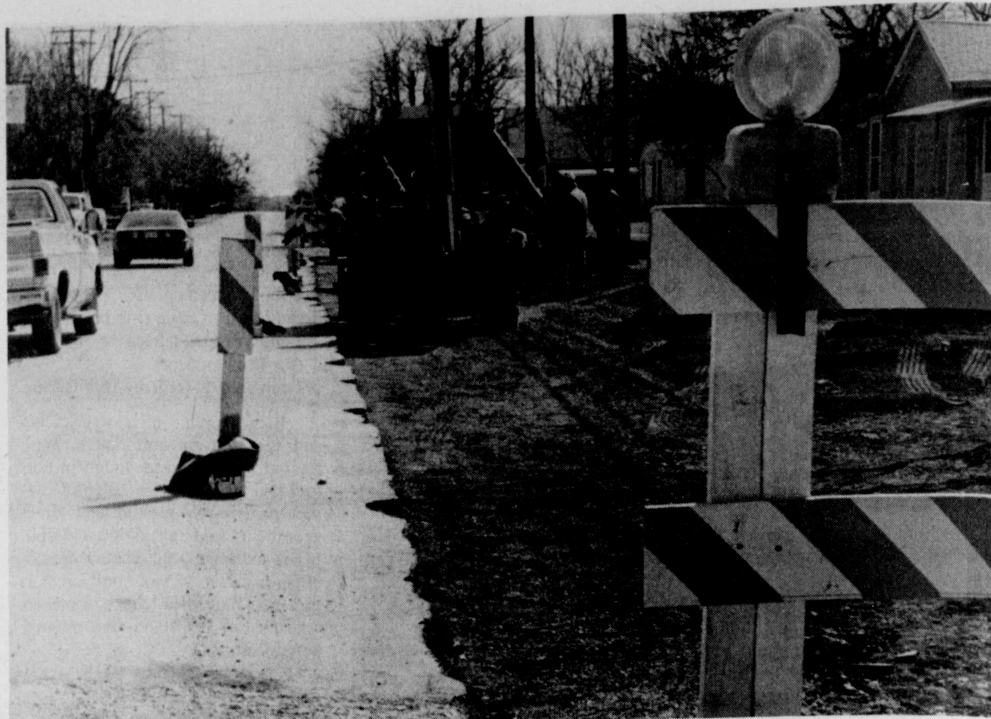
WORK IS UNDERWAY to reconstruct South Wall, as crews began widening the shoulder of the pavement. Driving will be inconvenient the next few months, according to contractor Terry Edwards, but the results will be easier, safer driving for years in the future.
