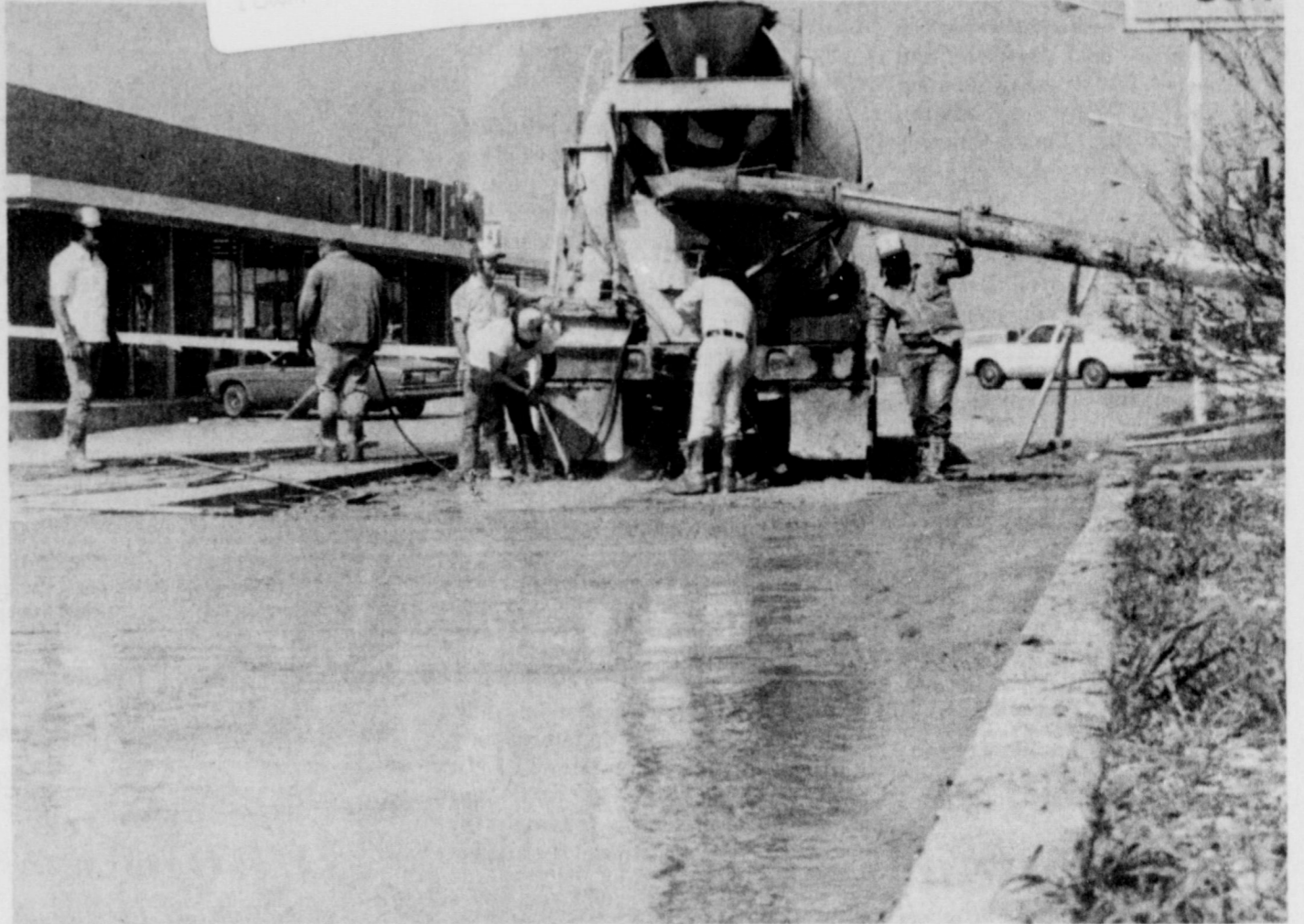
LAST SLAB POURED- Workers pour the final section of concrete paving Tuesday morning on West Park, completing a project which replaced paving so warped some
