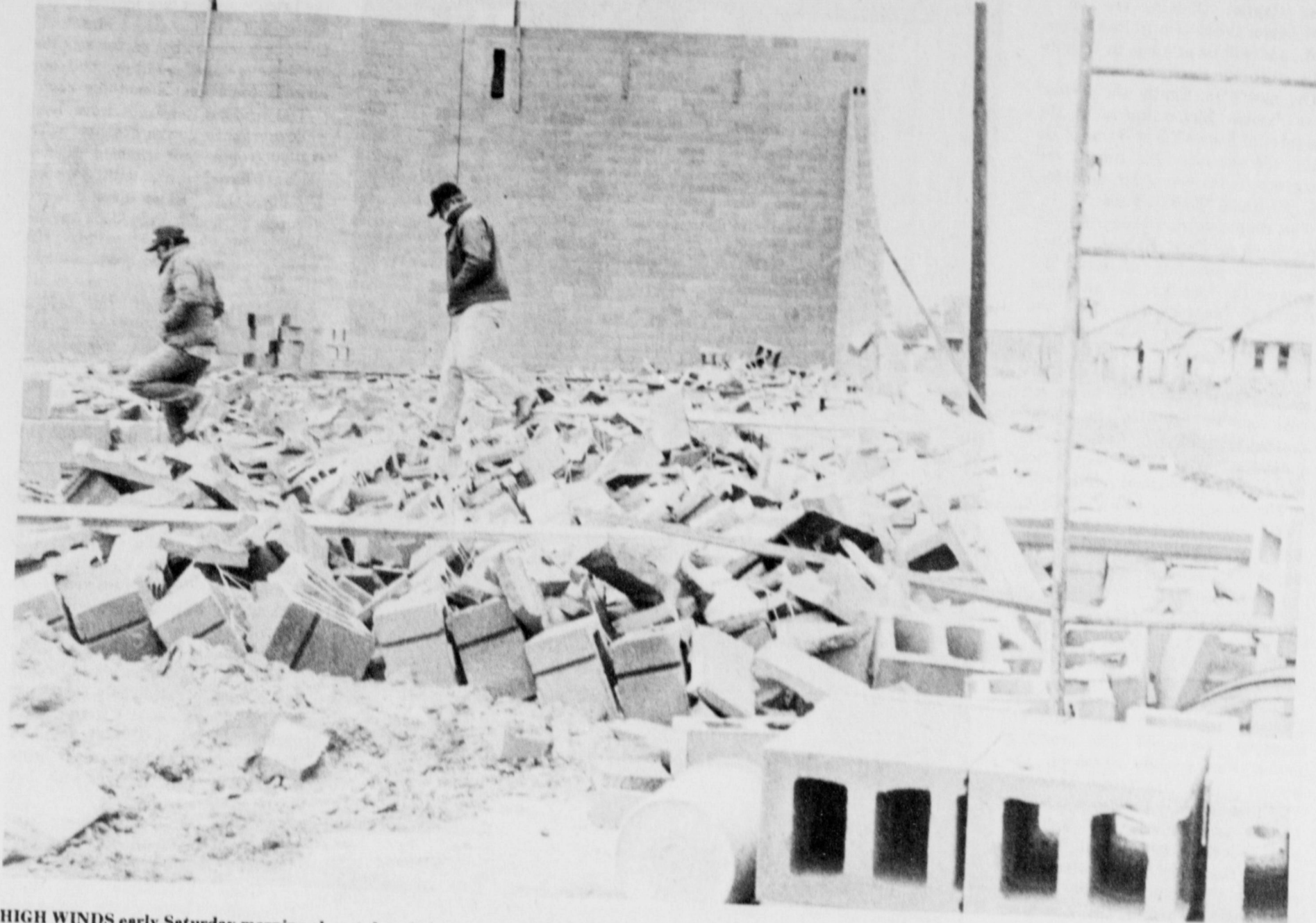
HIGH WINDS early Saturday morning almost demolished the north wall of the new Wal-Mart store. The wall had been built as high as the west wall, in the picture's background, and was braced, but not adequately to withstand
