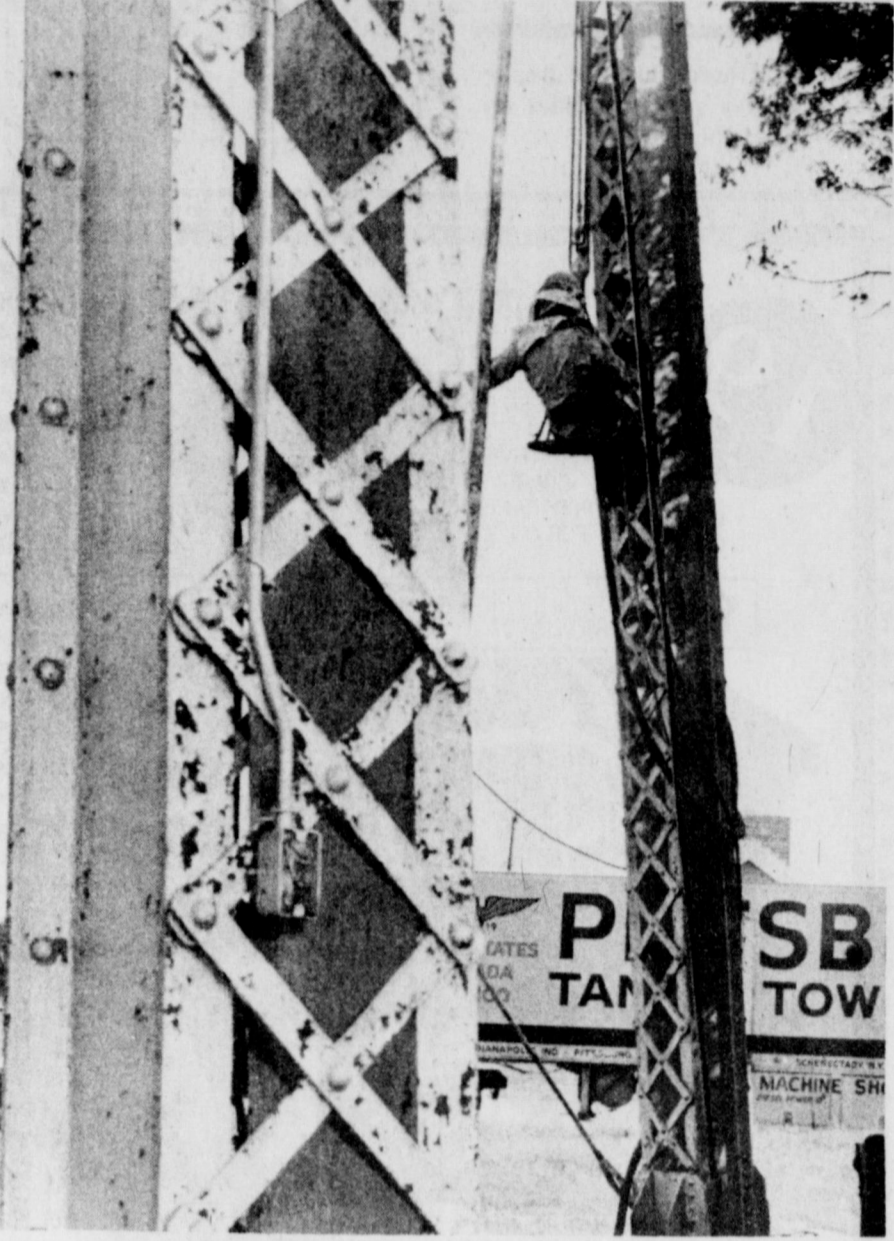
NOISE AND SANDY GRIT will continue in the neighborhood of the city hall and post office for a few more days, while workers continue sandblasting the old water tower. Like farmers, sandblasting work has been delayed by wet weather and high humidity. Painting will follow.
