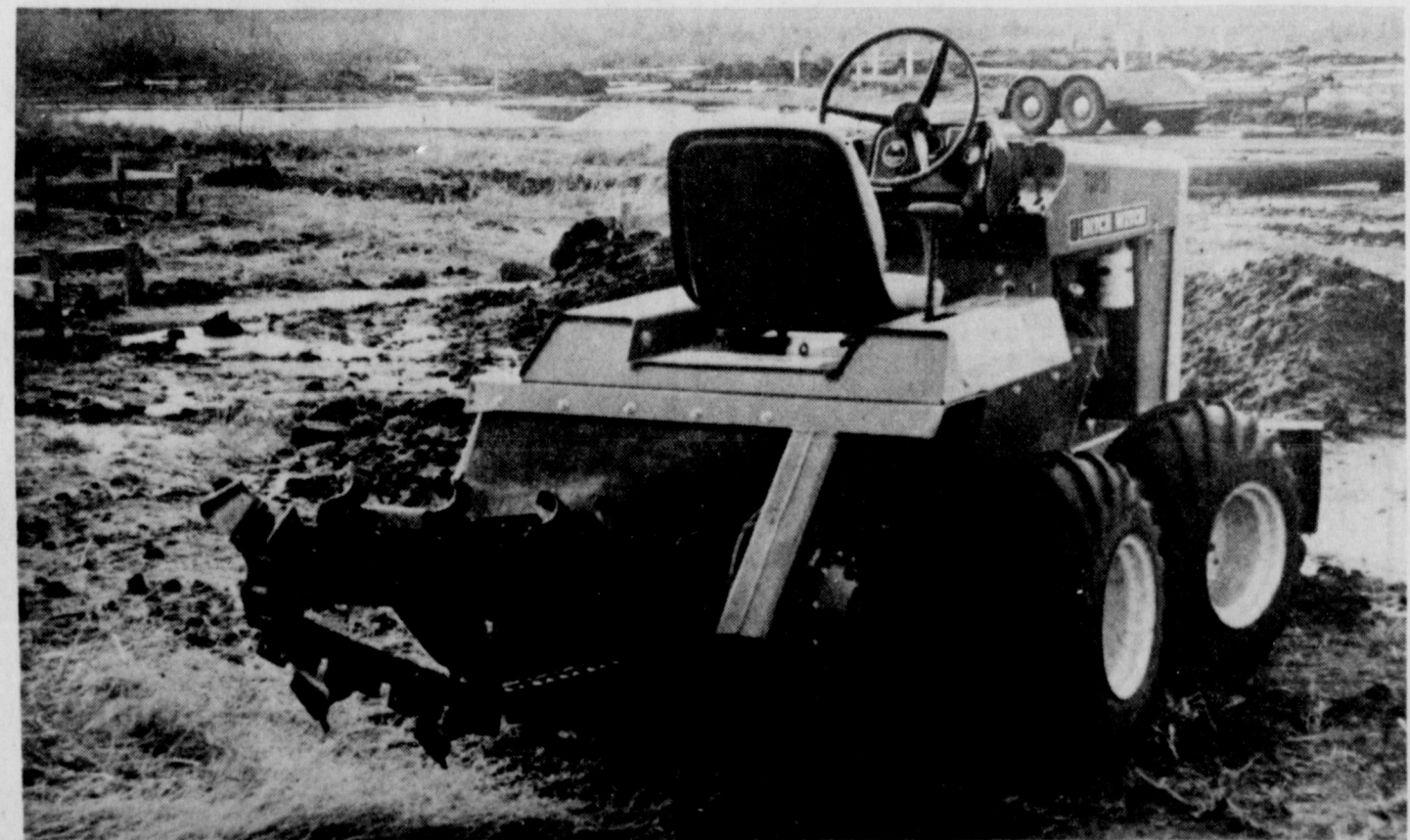
CONSTRUCTION on a new apartment complex in the south part of town, started late last week, was temporarily halted Tuesday by a rainstorm. The complex, located a
