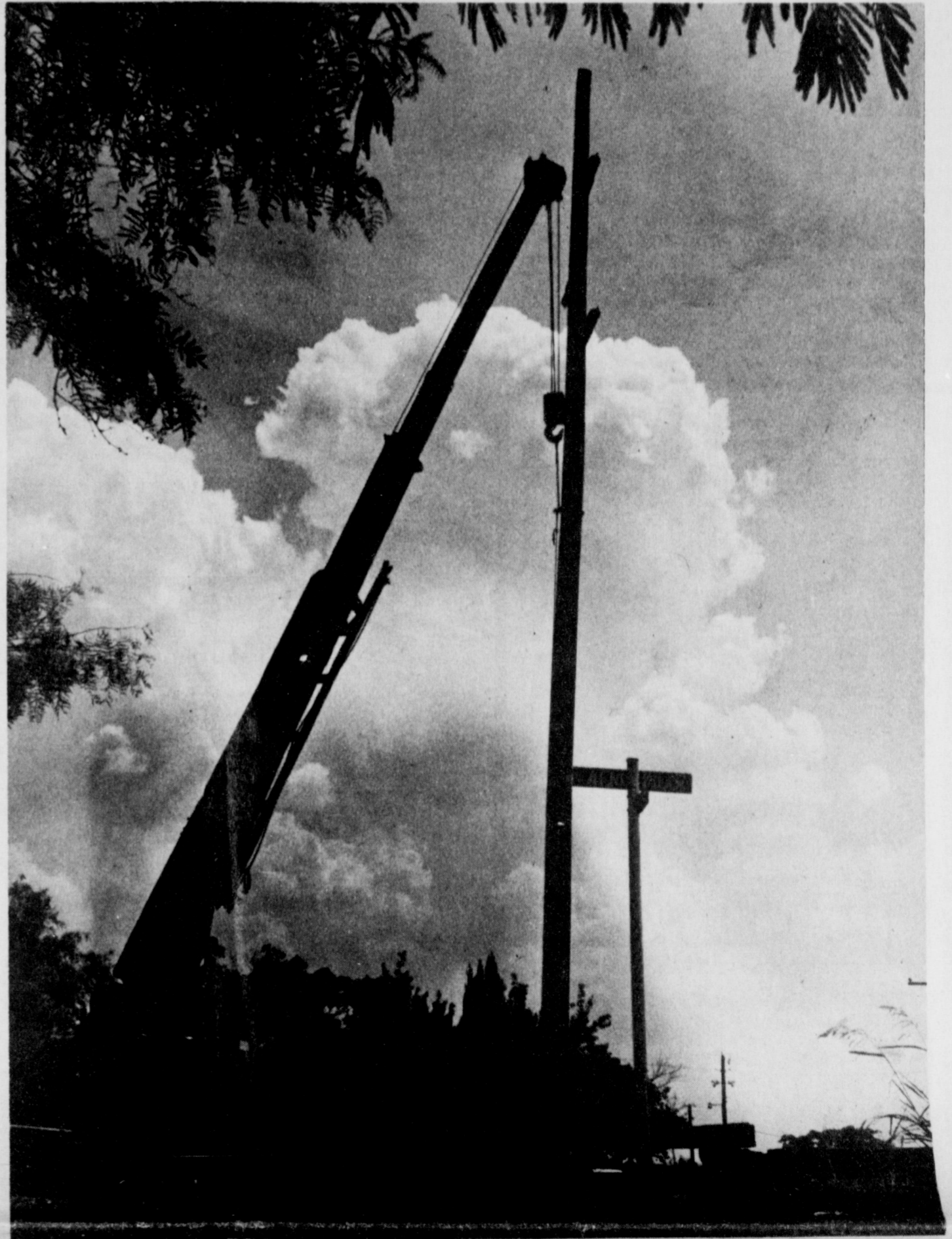
TOWERING POLES are being erected along West Magnolia which will allow Texas Electric Service Company to service Cryovac with 69,000 volts of electricity. The huge, 65-foot tall poles almost double the regular height poles throughout town. Line completion is expected this week, but it will not be energized until early August,
